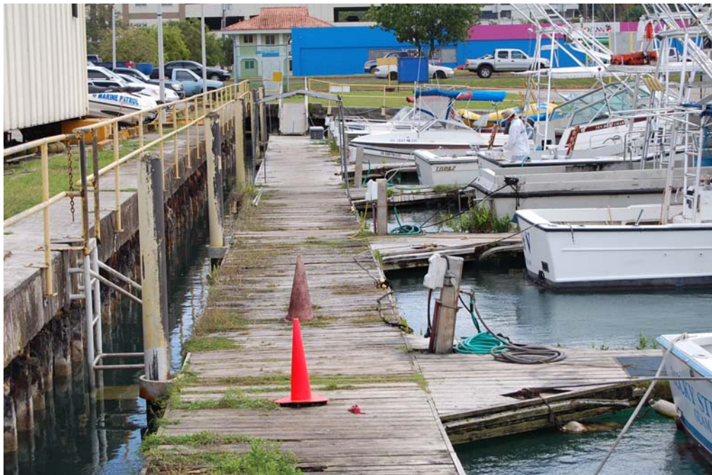
Southerly view along marina “A” Dock. Note the poor condition of the wood dock and rusting sheet piling. Dock and sheet piling improvements commenced in May 2011.
