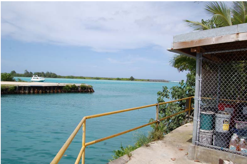
Northwesterly view across east and west breakwater from a point along east breakwater improvements.
