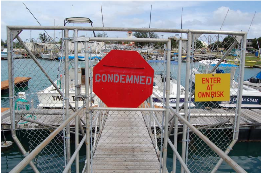
Easterly view at “condemned” dock area due to deterioration of improvements.
