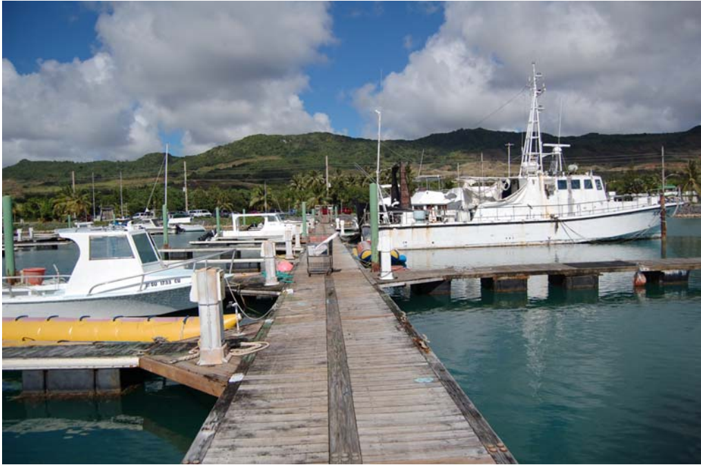
Easterly view along typical dock. Note the poor condition of the dock and the slips.
