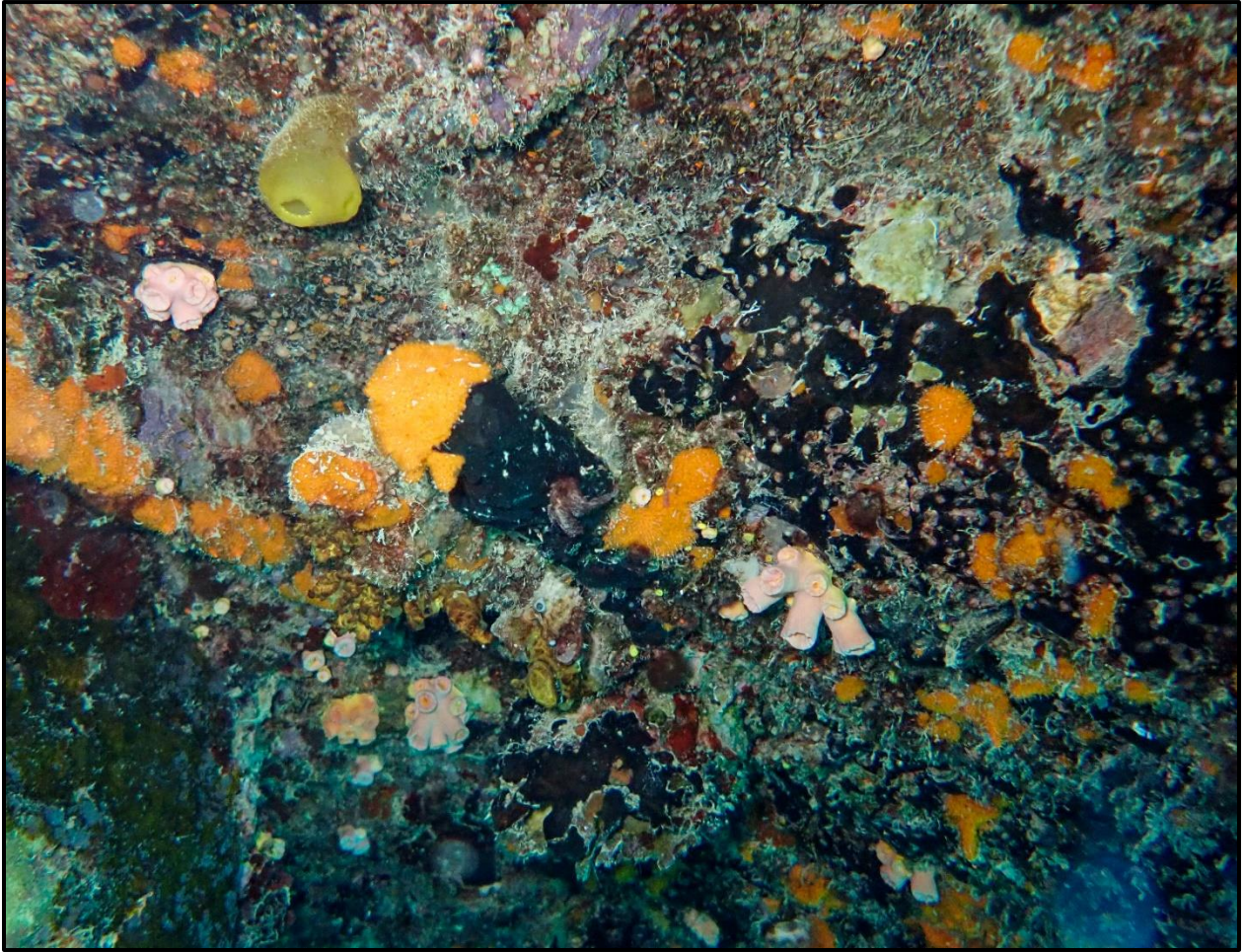
Figure 26. A benthic community dominated by encrusting sponges and turf algae, and numerous dendrophylliid corals, typical of the underside of the concrete beam that extends across the length of the wharf sides at a depth of approximately 1.5 m.
