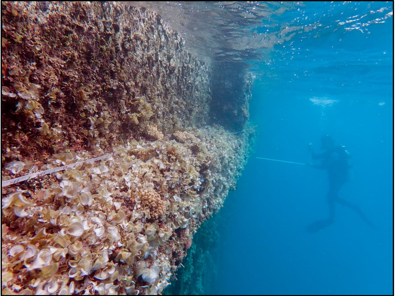
Figure 23. One of the shallow (~1.5 m) transects placed on a concrete beam that runs the length of the wharf sides.
