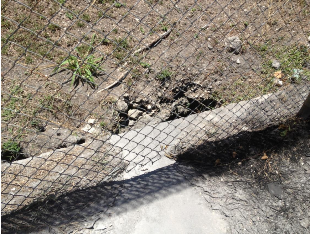
Photo Description: Sinkhole along pavement edge.
