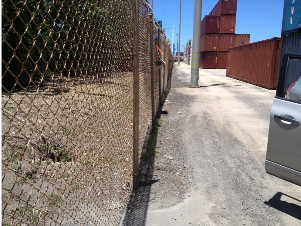
Photo Description: Sinkholes along the southern fence south of the container terminal gate administration building looking west.
