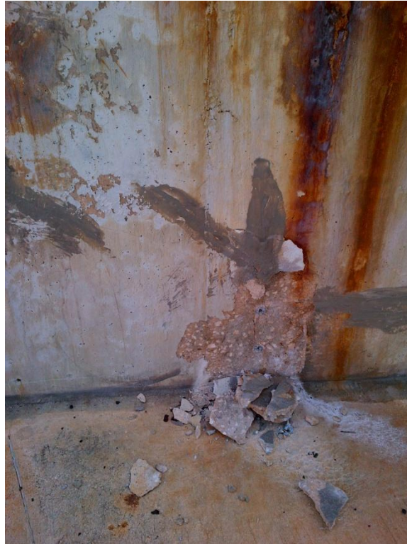
Photo Description: Spalling on the northern retaining/ containment wall.
