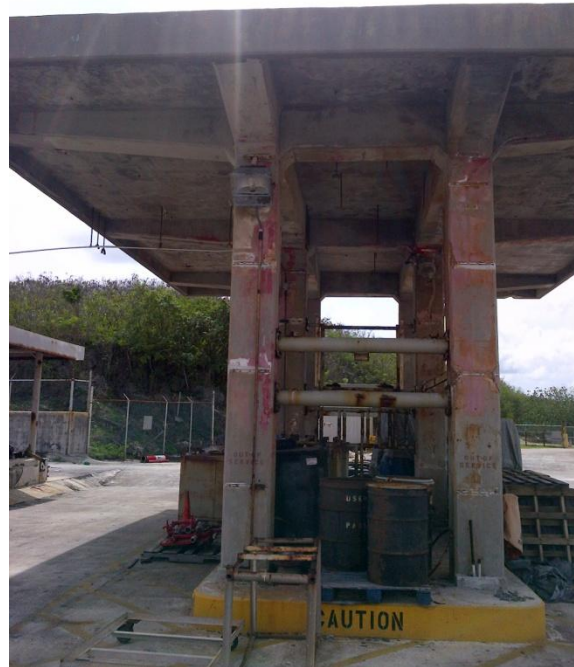
Photo Description: Loading rack structure located south of the pump shelter looking east. The piping has been removed from the structure.
