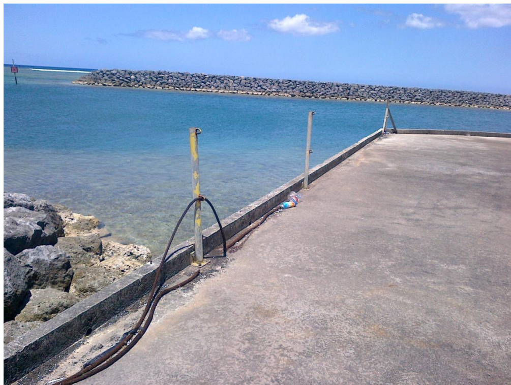
Photo Description: South edge of elevated pier looking west towards marina breakwater.
