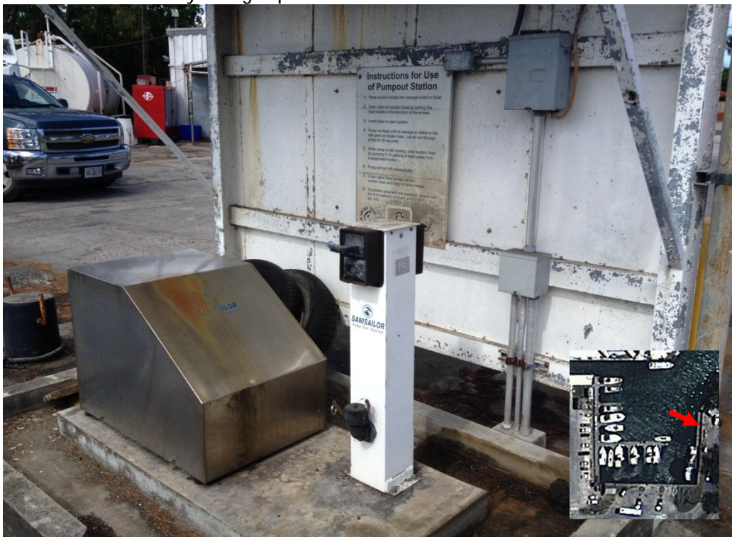
Photo Description: Waste pumpout station located near fuel pumps on eastern side of east basin of the marina.
