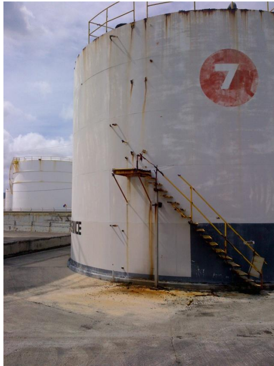
Photo Description: Tank 7 looking southeast from western ramp. The ladder and fill height indicator are both missing. Tank is out of service.
