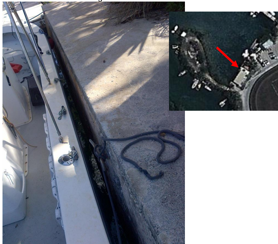
Photo Description: Sheetpile concrete in good condition. Sheet pile was not visible.
