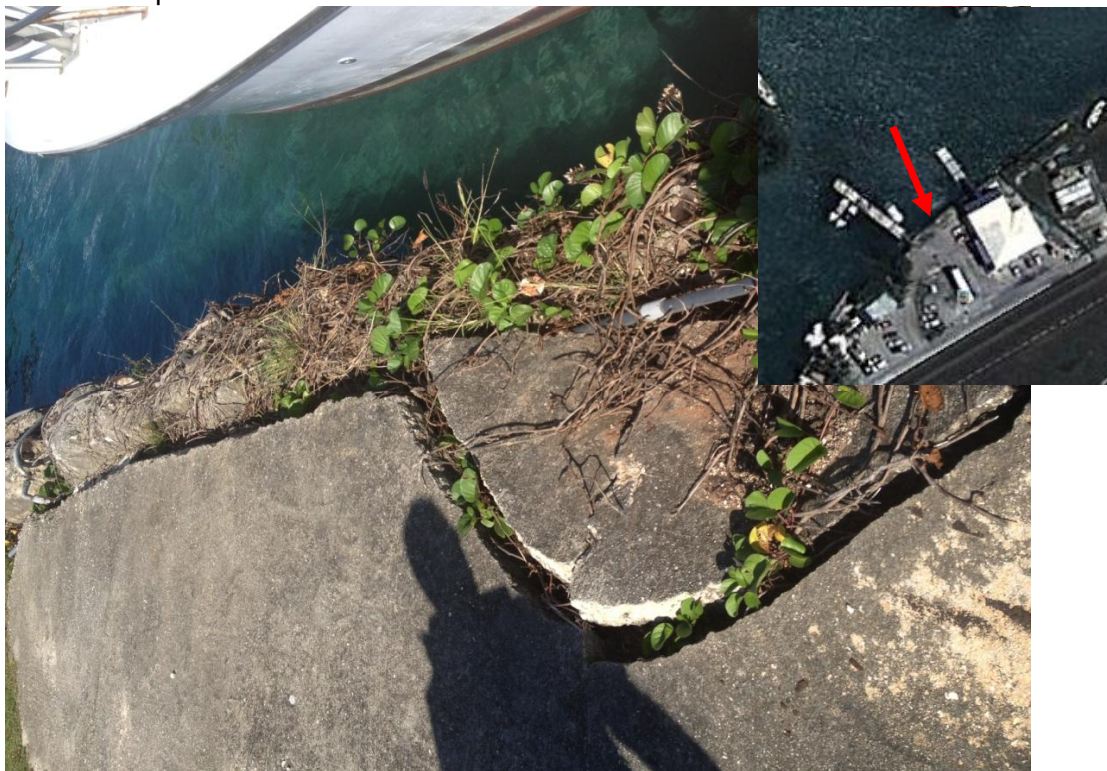
Photo Description: Sink hole forming behind bulkhead near Aqua World on the northern edge of the parking area.
