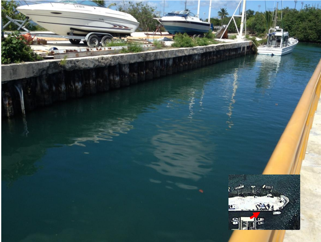
Photo Description: Northern sheetpile wall of the boat basin looking northeast from the center peninsula.
