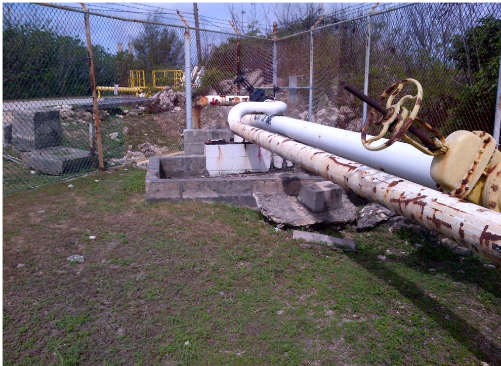
Photo Description: Abandoned pipelines that connected Tank Farm A to Golf Pier along the eastern perimeter fence looking southwest towards the 'wye' from golf pier.
