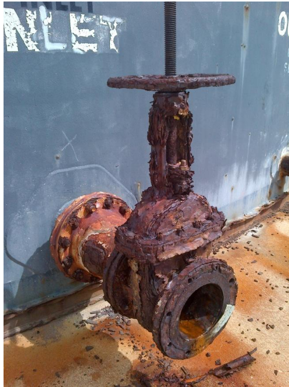
Photo Description: Tank 3 inlet valve on the eastern side of the tank.
