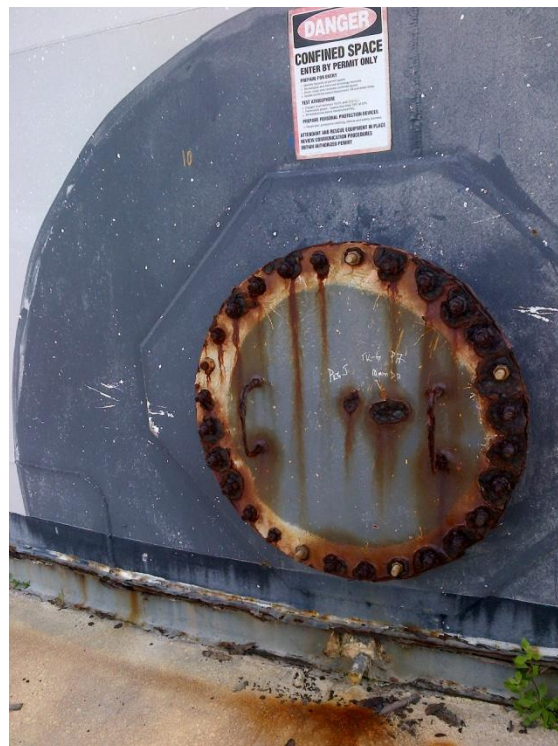
Photo Description: Access flange on tank 6 on the eastern side of the tank looking west.
