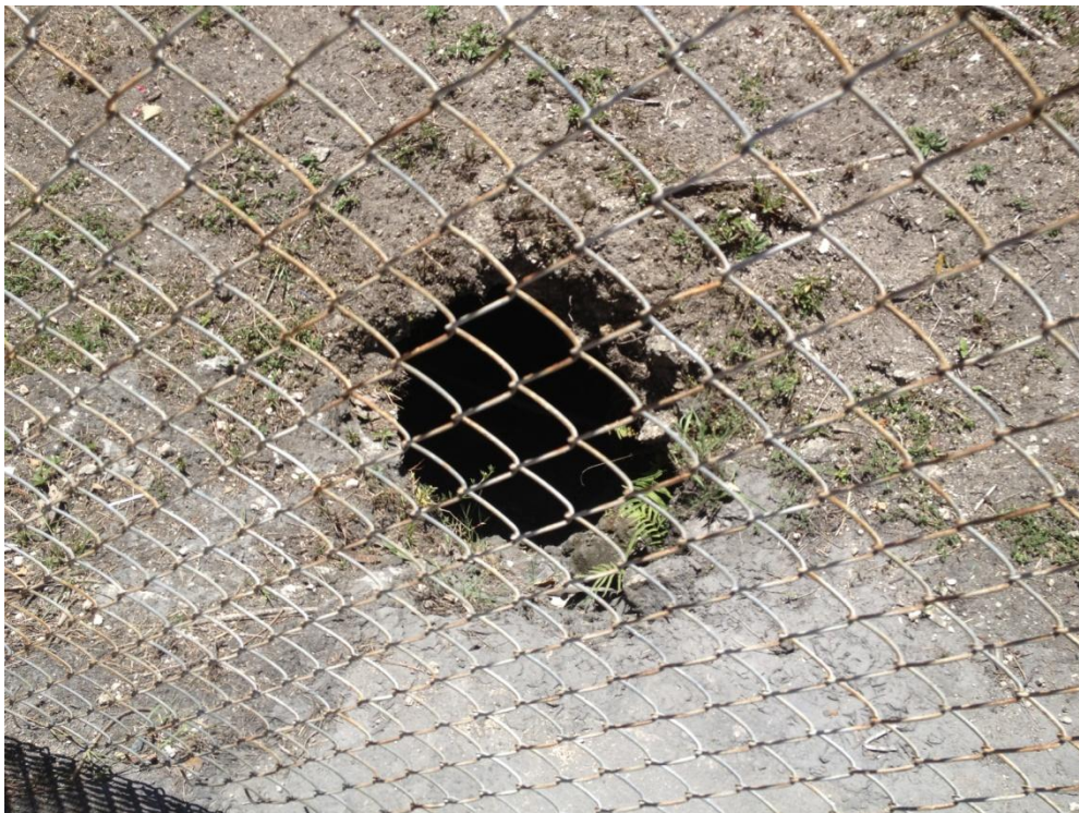
Photo Description: Sinkhole along pavement edge.
