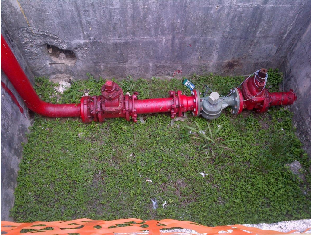
Photo Description: Domestic water supply line to Golf Pier.
