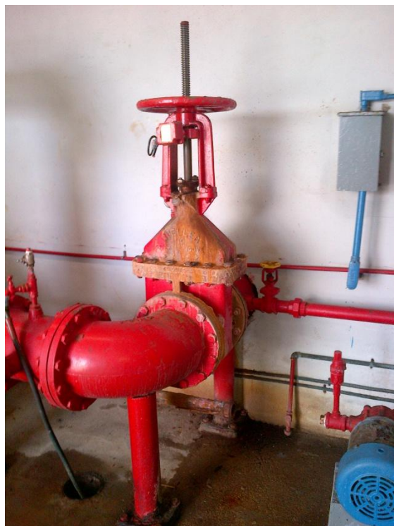
Photo Description: Freshwater fire pump piping.
