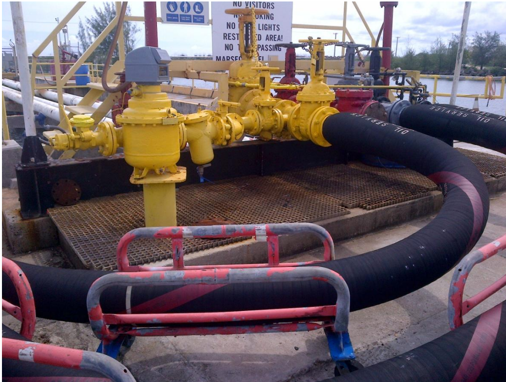
Photo Description: Valves and hoses on the Golf Pier structure.
