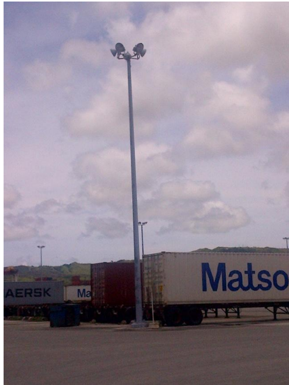
Photo Description: Container yard lights installed in 2012 in the eastern portion of the yard looking southeast.
