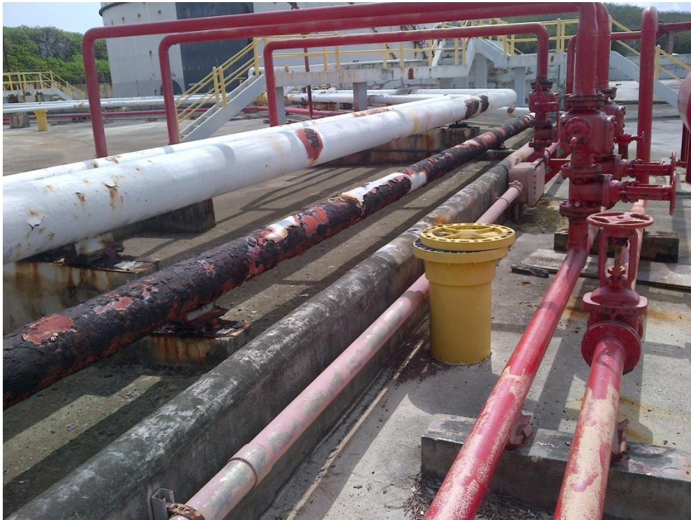
Photo Description: Abandoned pipelines running through the center of the yard. Looking northeast towards tank 1.
