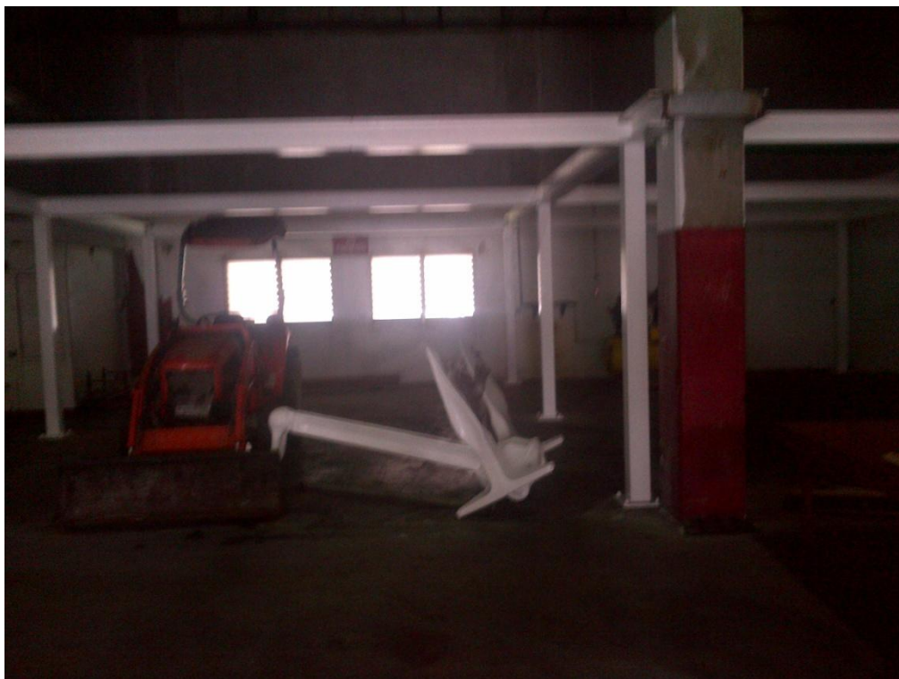
Photo Description: Steel frame within EQMR Building facing north. The frame should be disconnected from the building columns for seismic considerations as the current situation would impose additional stress to the existing structure.
