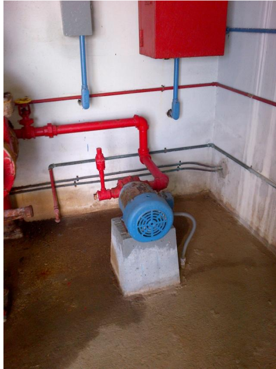
Photo Description: Freshwater jockey pump in the fire pump building. The jockey pump was not working during the assessment.
