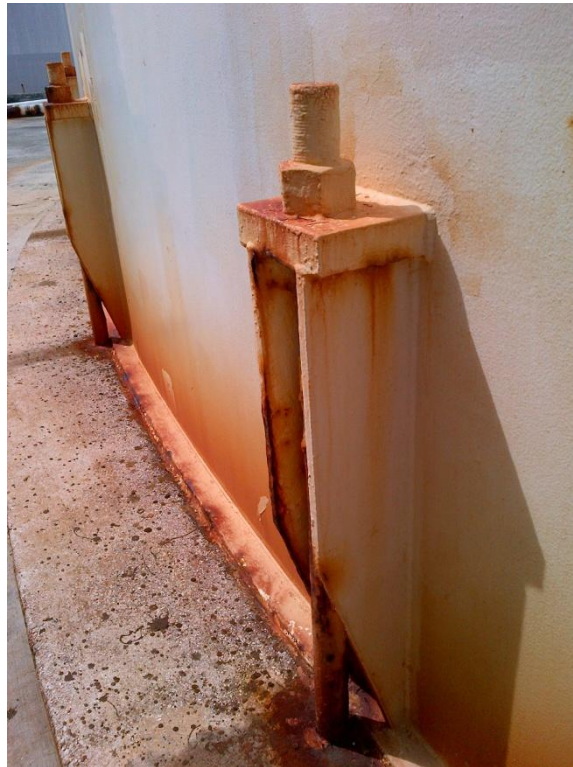
Photo Description: Tank 2 anchor bolts on the north side of the tank.
