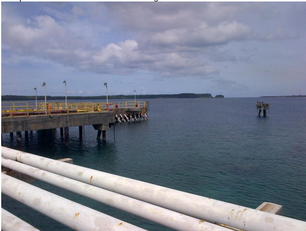
Photo Description: Breasting and mooring dolphins to the west of the Golf Pier main structure.
