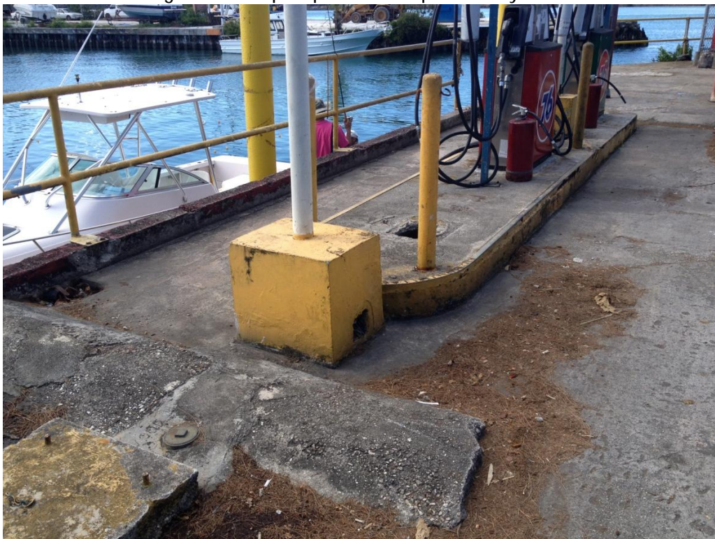
Photo Description: Containment perimeter around Fuel Island should be addressed by the operator.
