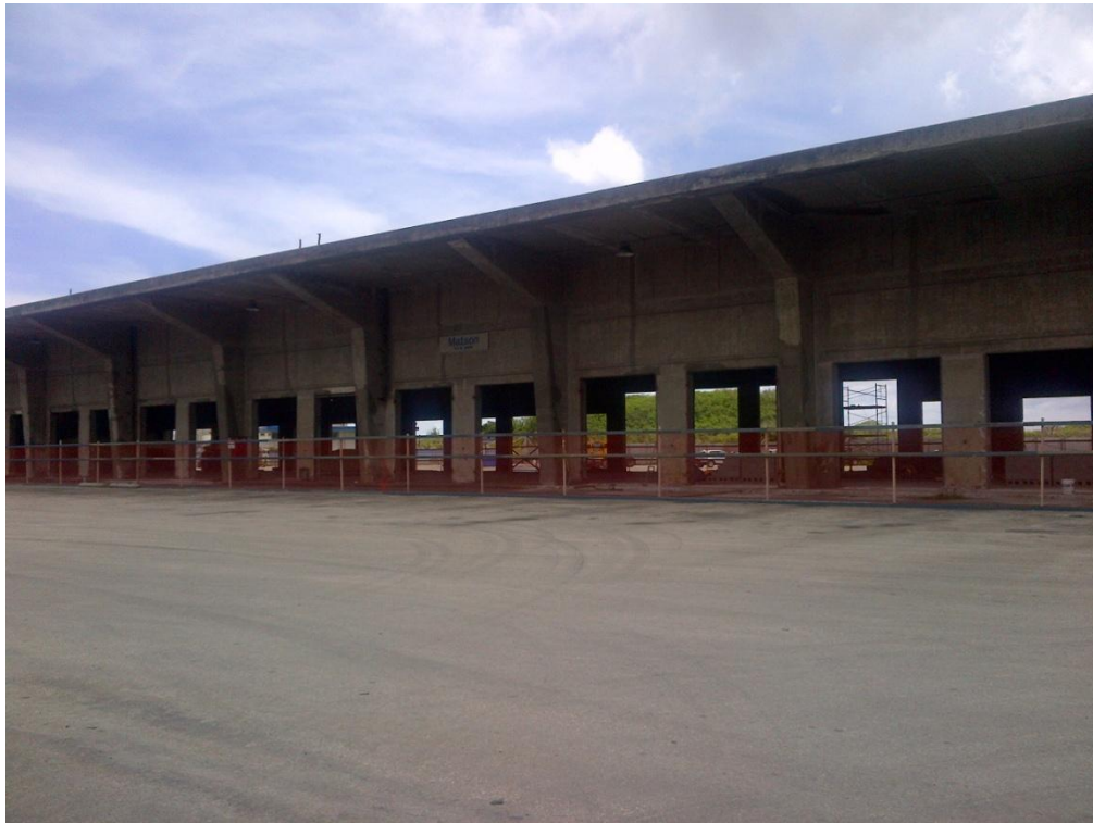
Photo Description: CFS Building stripped and ready for renovations by the MarAd Program looking northwest.
