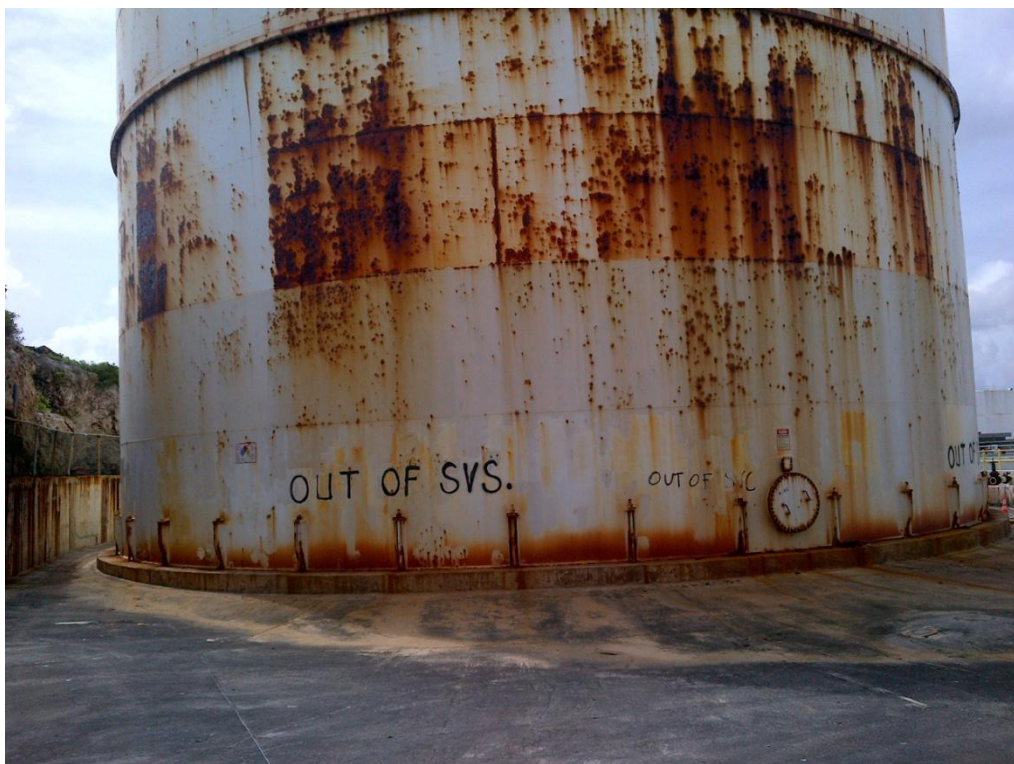
Photo Description: Tank 2 looking east. The tank has been disconnected and is out of service.
