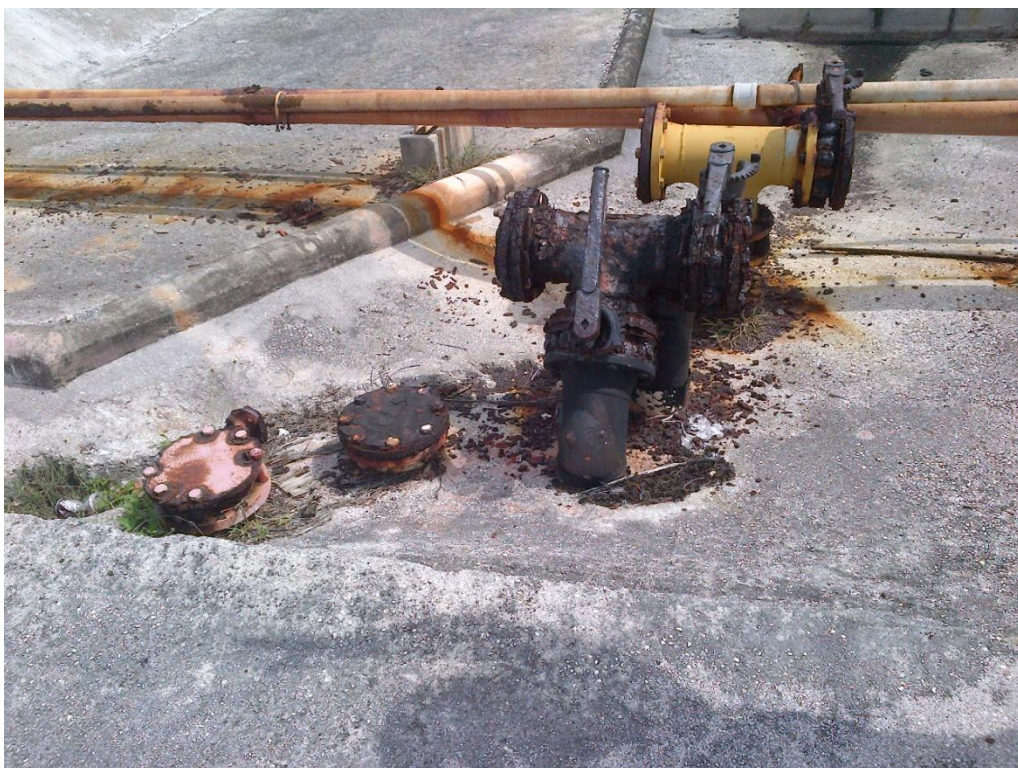
Photo Description: Underground piping that connects the loading rack to the pipelines in the site.
