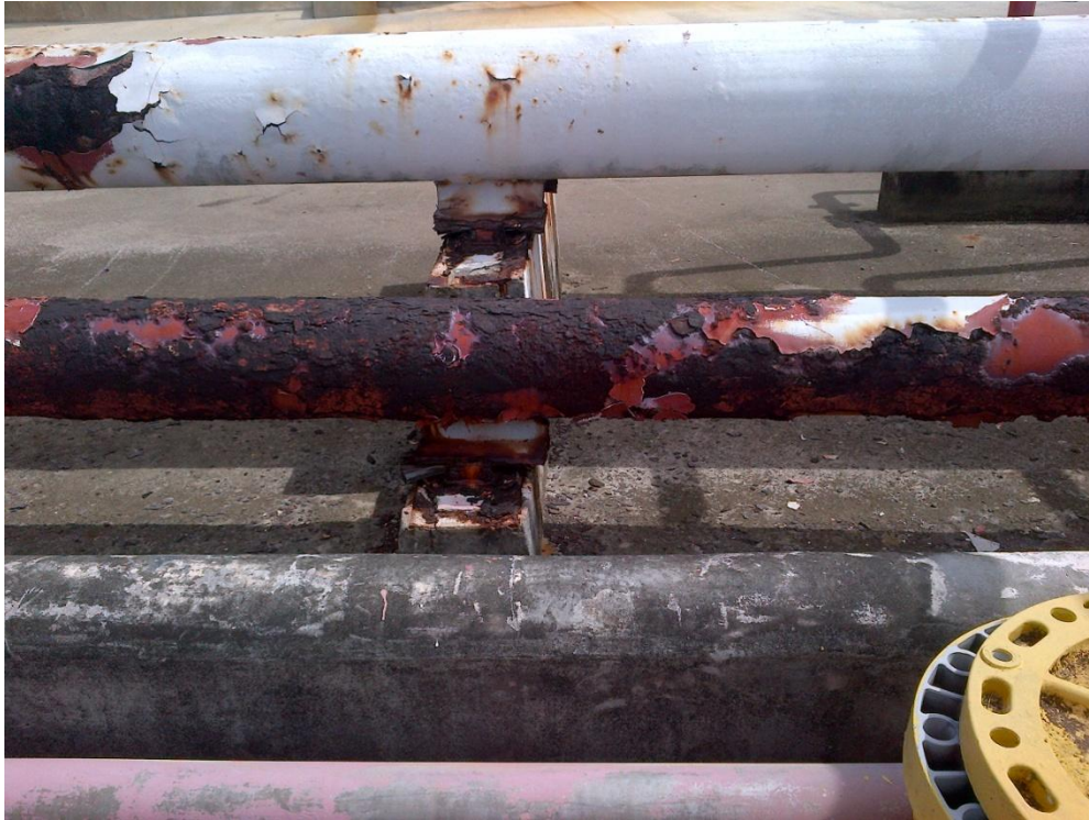
Photo Description: Abandoned pipelines in the center of the tank farm. The piping is in very poor condition for what is remaining. A fair amount of the piping has been removed on the north end of the site.
