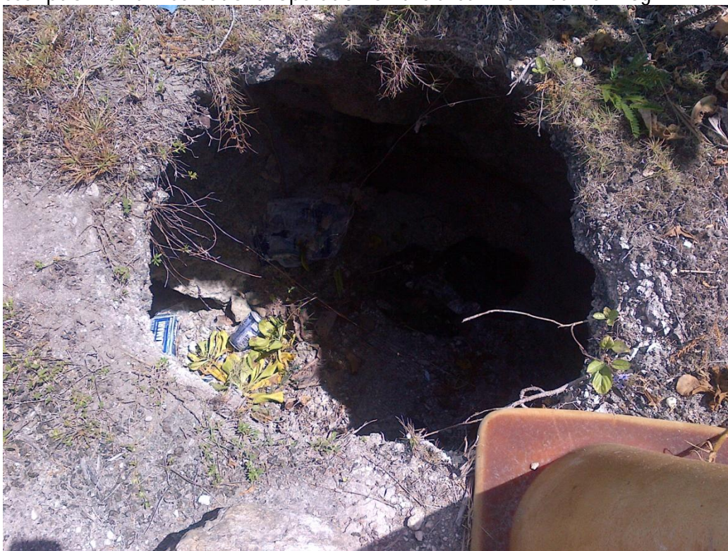
Photo Description: Sink hole on the shoulder of the access road between Hotel Wharf and Golf Pier.
