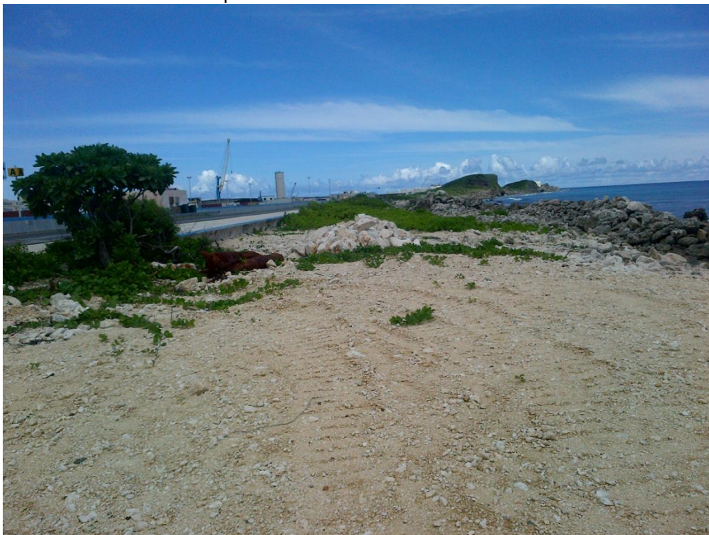
Photo Description: DPW Seawall project looking west from the ending point. The area west of the Gate Administration Building was not completed.
