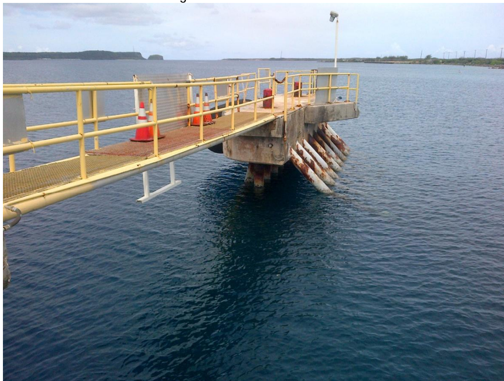
Photo Description: Western breasting dolphin and associated catwalk from the Golf Pier main structure.
