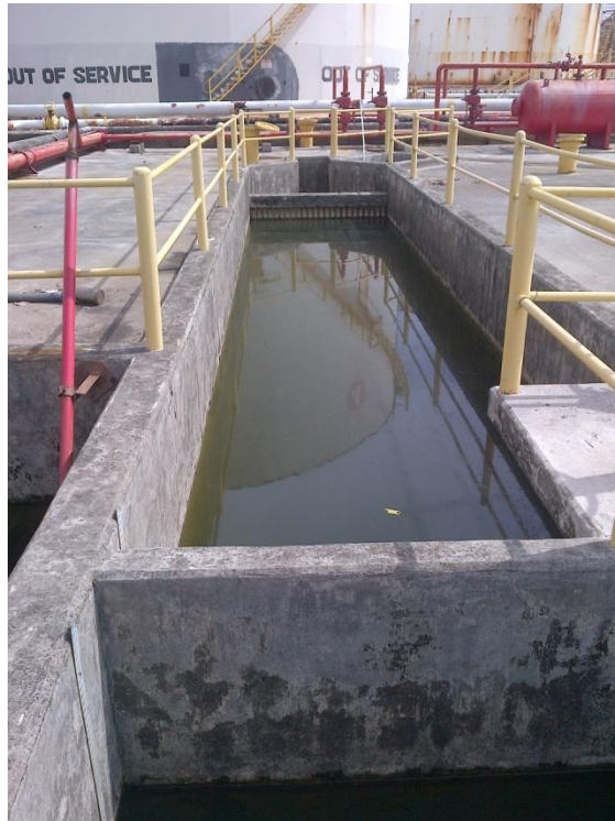
Photo Description: Oil water separator east of tank 6 looking north towards tank 4. Directly south is the fire pump house.
