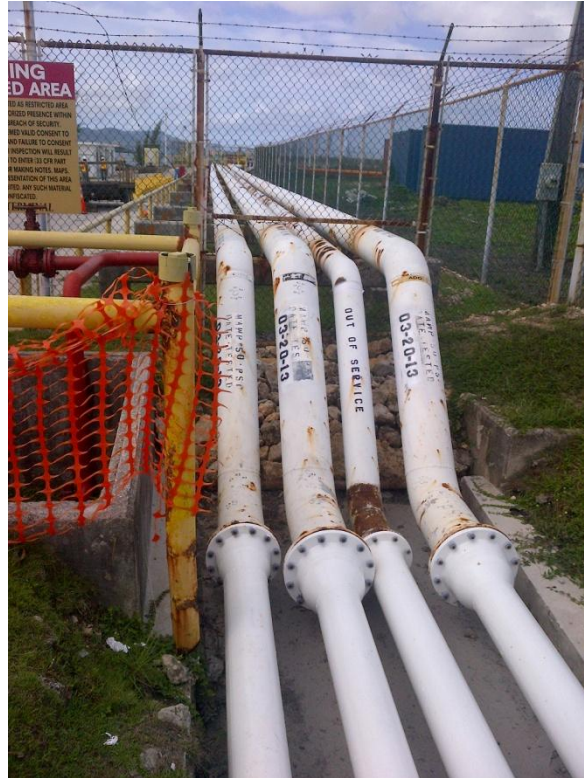
Photo Description: Fuel lines entering onto Golf Pier looking south.
