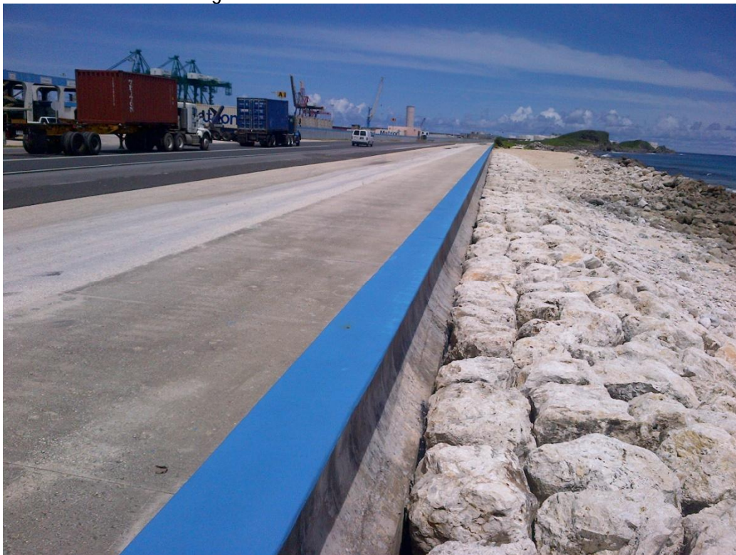
Photo Description: DPW Seawall project looking west at the Gate Administration Building.
