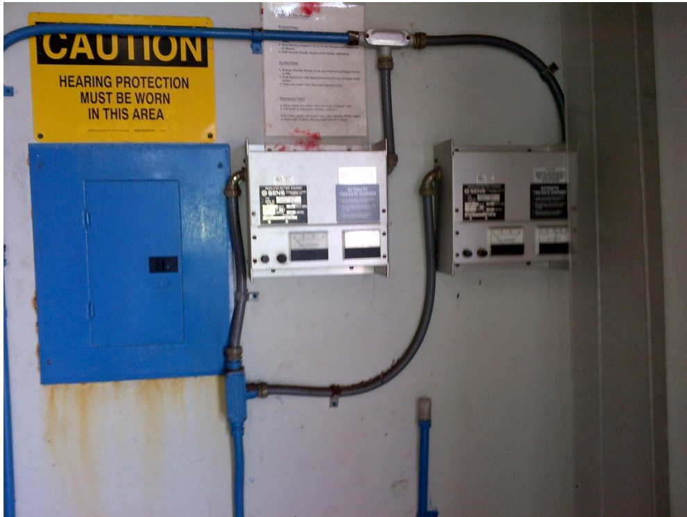
Photo Description: Diesel fire pump battery chargers/ maintainers on the eastern wall of the pump building.
