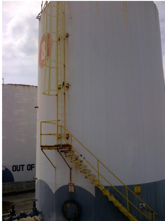
Photo Description: North side of tank 8 looking southeast. The ladder appears to be in good shape with slight rusting. The stairway needs cleaned and repainted. The fill height indicator is missing from this tank.
