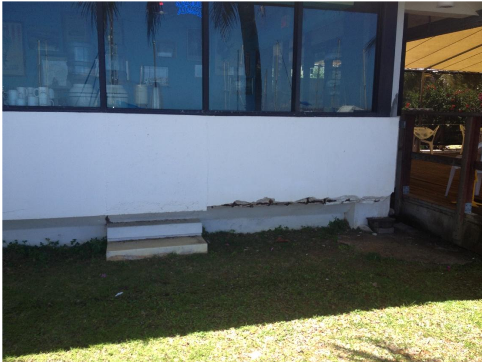
Photo Description: Southern end of western wall of restaurant building has spalling along the drip line.
