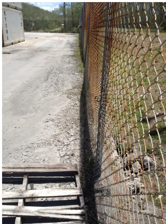
Photo Description: Sinkholes along the southern fence south of the container terminal gate administration building looking east.
