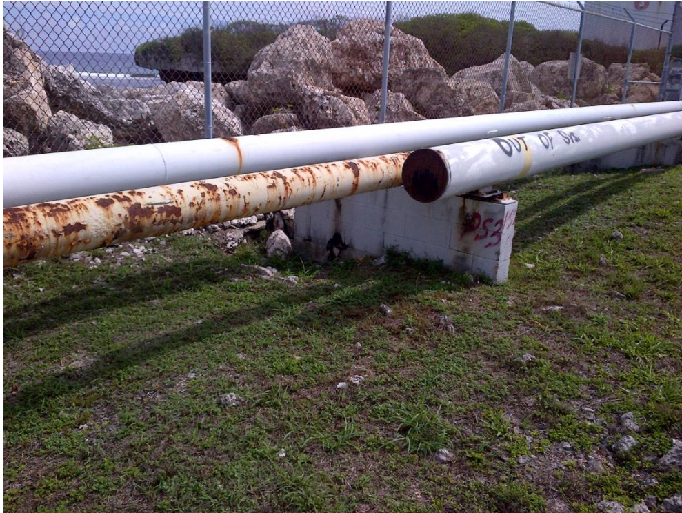
Photo Description: Abandoned pipelines that connected Tank Farm A to Golf Pier along the eastern perimeter fence looking north.
