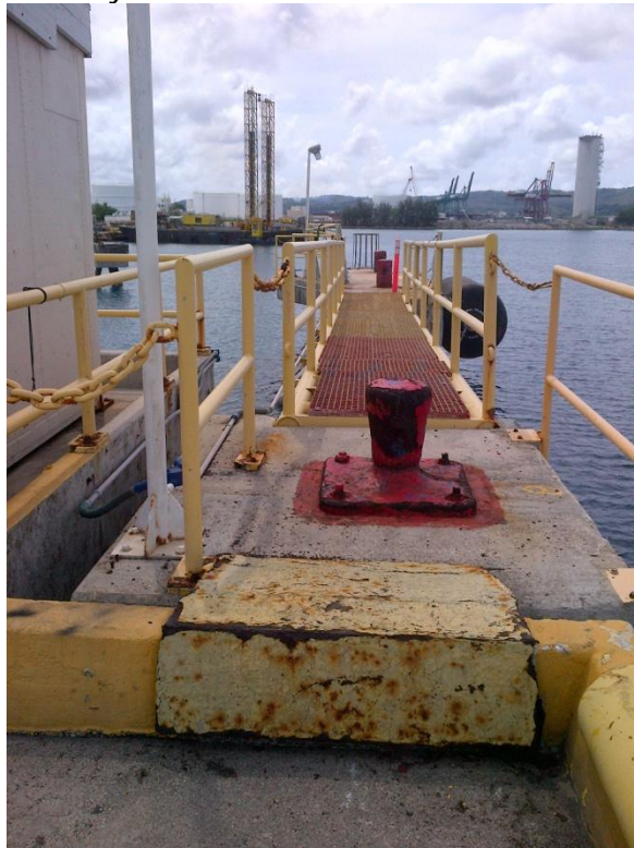
Photo Description: Catwalk to the breasting dolphin to the east of the Golf Pier main structure.
