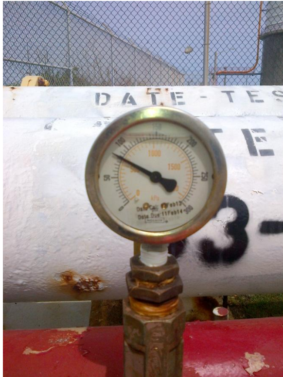
Photo Description: Domestic line at static pressure of roughly 80psi.
