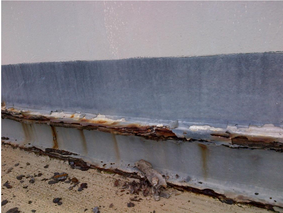
Photo Description: Rust has penetrated the floor of tank 6. The flakes were coming out from under the tank wall.
