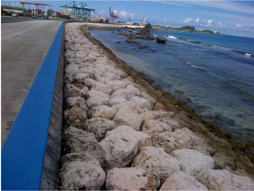
Photo Description: DPW Seawall project looking west towards the Gate Administration Building.
