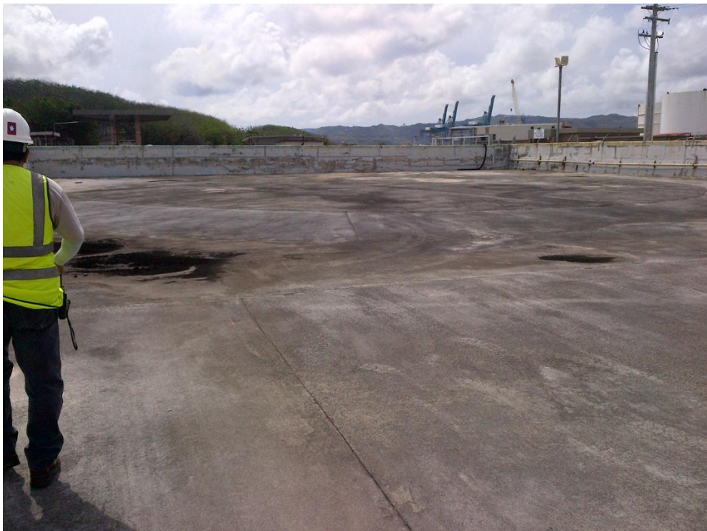
Photo Description: Site location where tank 5 was before being removed. The containment perimeter is in good condition.
