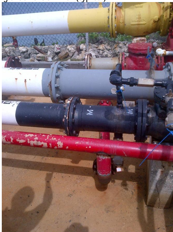
Photo Description: Cross over pipe from a converted fuel line that supplies water from the fire pumps in tank farm A and C to Golf Pier.
