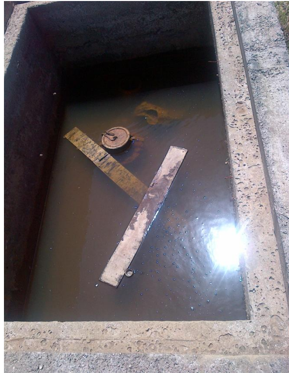
Photo Description: Water Service Pit on Hotel Wharf.
