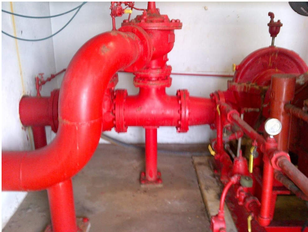
Photo Description: Freshwater fire pump piping in the west half of the pump building.
