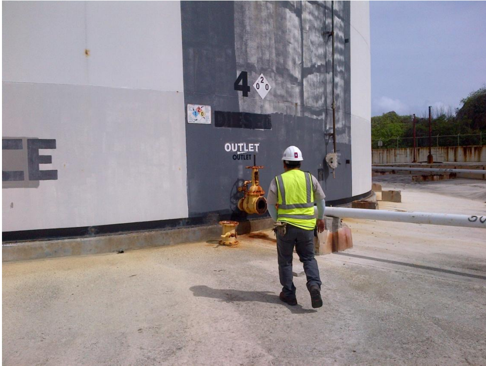
Photo Description: Tank 4 looking from the center of the site to the northwest. The tank has been disconnected and is not in service.
