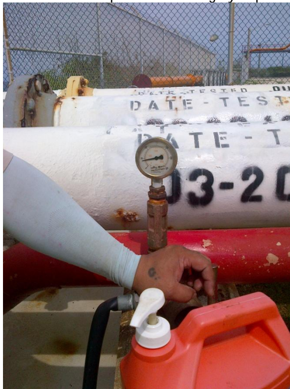
Photo Description: Pressure drops to 40 psi with a hose bib open.
