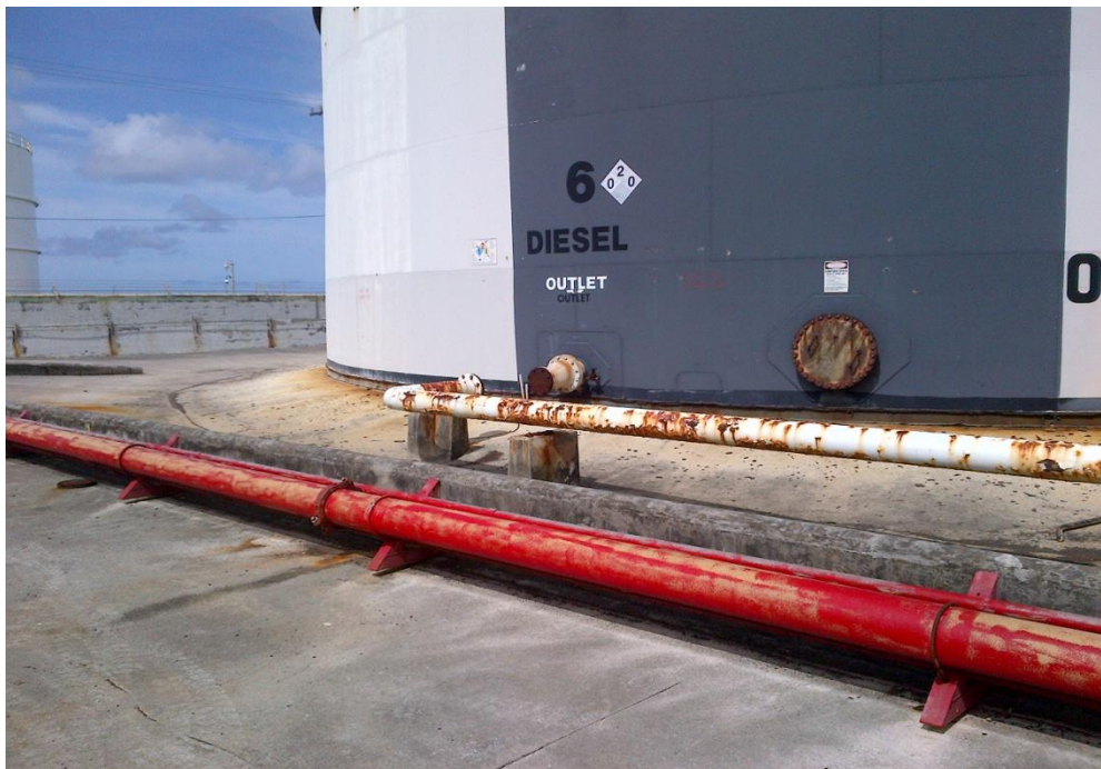
Photo Description: Looking southwest at tank 6. Fire supply line coming from the pump building from the left of the picture. Tank 6 has been disconnected and is not in service.
