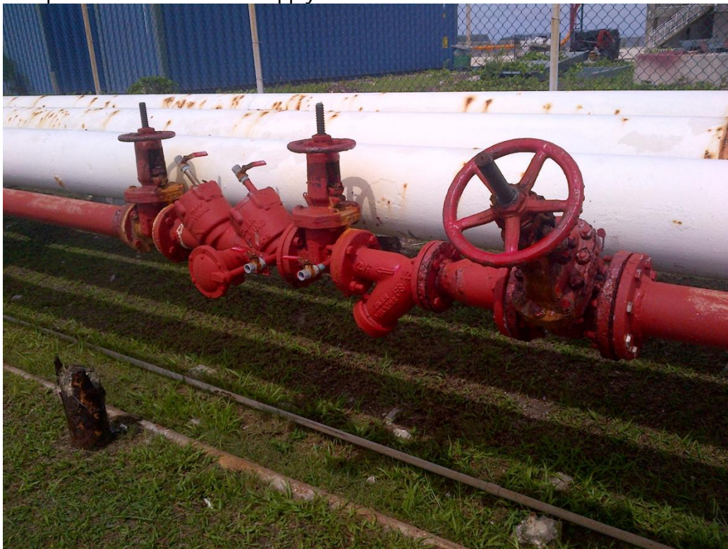
Photo Description: Backflow preventer and valves on the domestic water supply line. The main valve on the right is closed before engaging the fire pumps.
