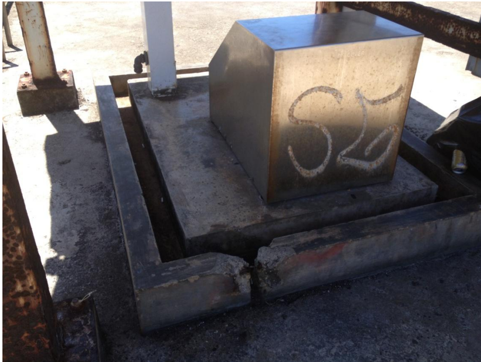
Photo Description: Pumpout station on elevated pier.
