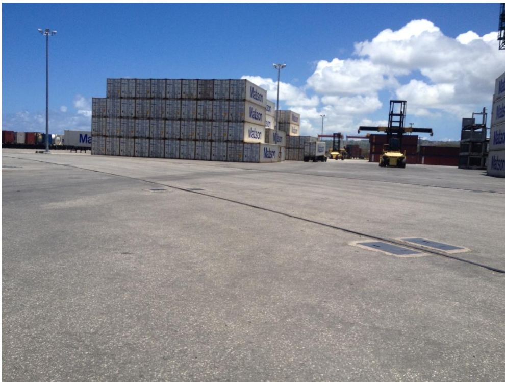
Photo Description: Asphalt paving in the central portion of the yard looking east. The gantry spur rail is centrally located in the photo.
