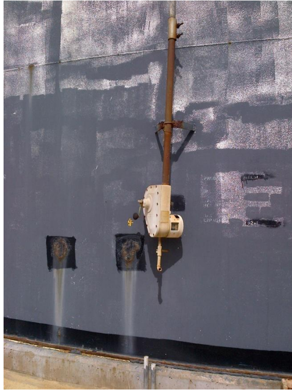
Photo Description: Tank 4 fill indicator. The tanks have been out of service so it is unknown if this works.
