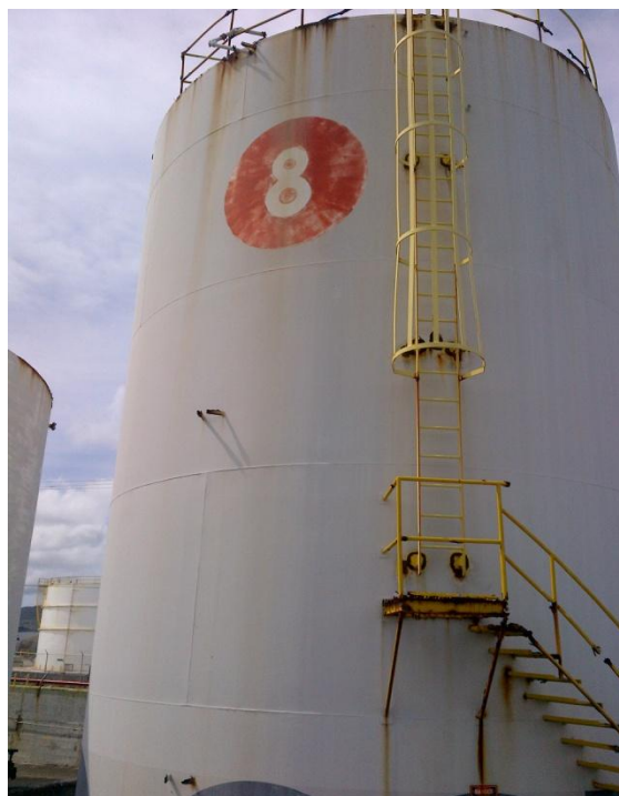
Photo Description: Closer look at tank 8 looking south from western ramp. Tank is used for storage of freshwater for the fire pump.
