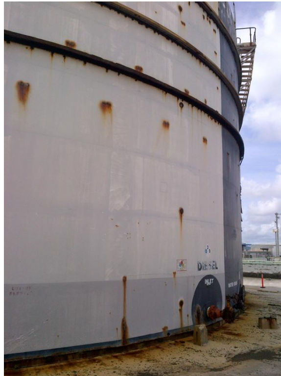
Photo Description: Tank 1 southern wall and stairway looking east. The tank is disconnected and out of service.
