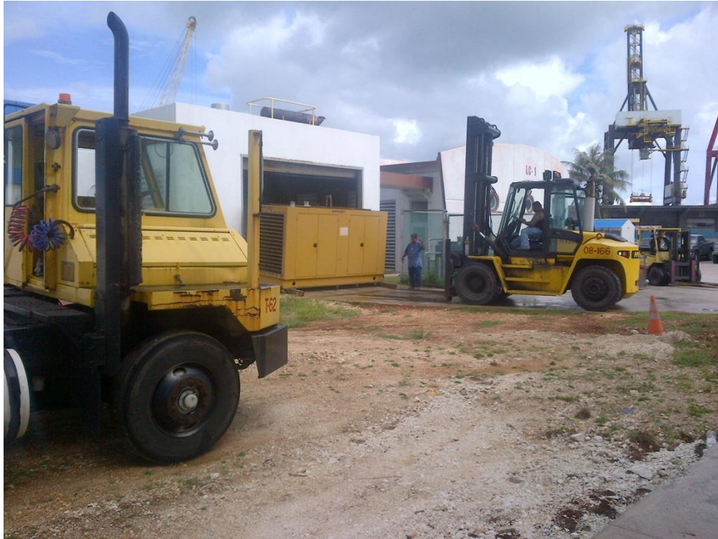
Photo Description: LC1 Generator building looking southeast. Generator is being removed and relocated to LC4.
