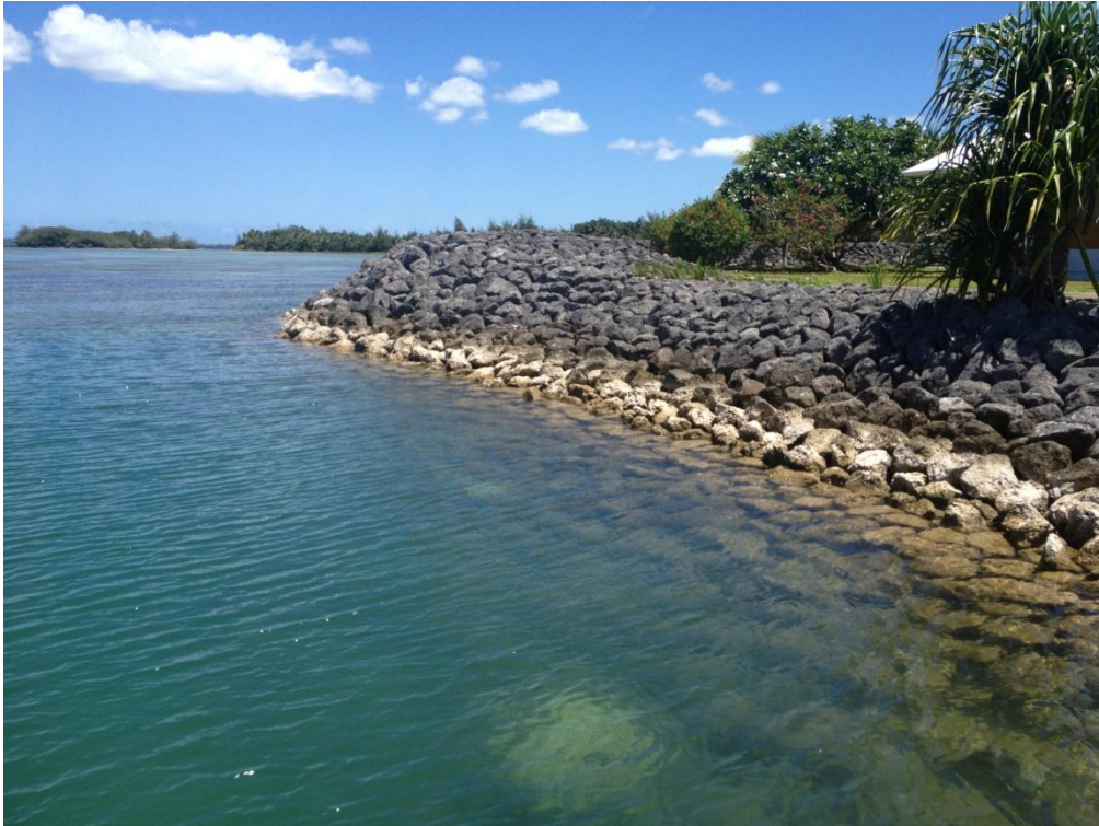
Photo Description: Looking north at the riprap shoreline at the northern edge of the marina.
