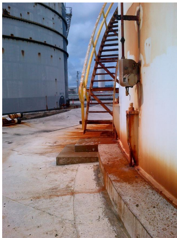
Photo Description: Tank 2 stairway on the south side of the tank looking west. Tank 4 is in the left edge of the picture.
