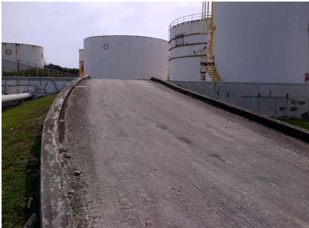
Photo Description: Western ramp into the tank farm looking northeast. Tank 8 is on the right of the frame with Tank 6 visible behind it. Tank 4 is in the middle and 3 to the left.
