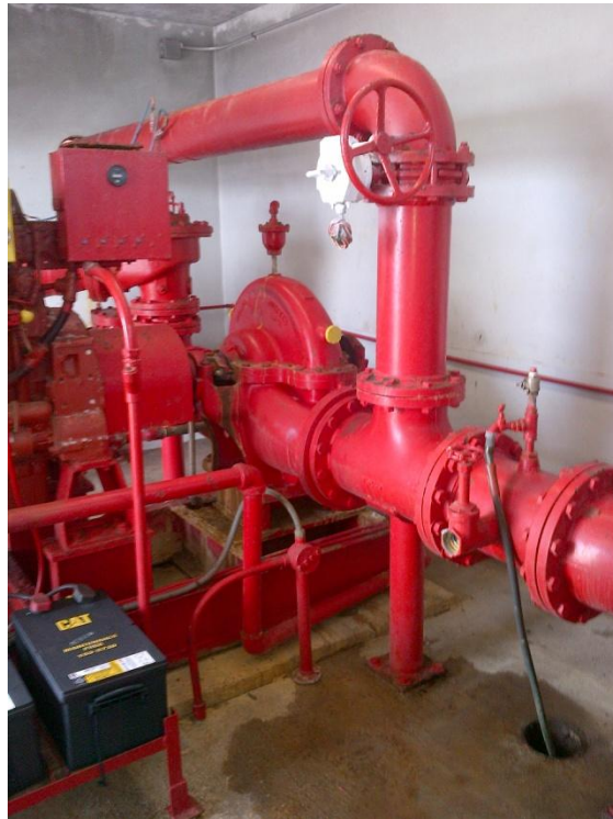
Photo Description: Freshwater fire pump piping on the east half of the building looking northwest.
