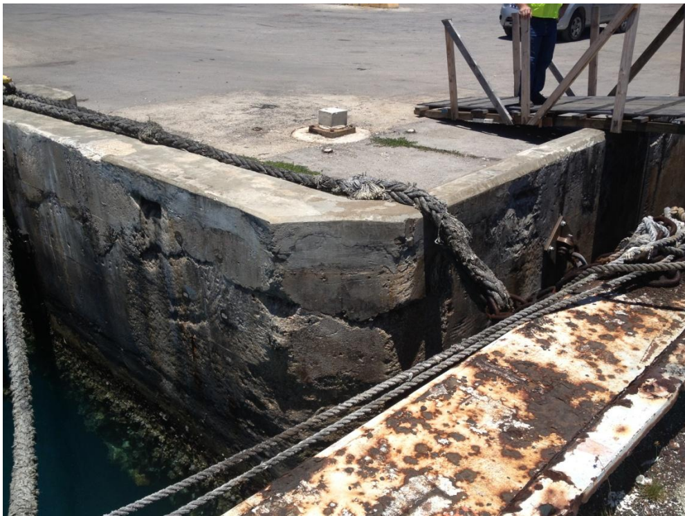
Photo Description: Concrete bulkhead corner at the end of F-6 looking northwest.
