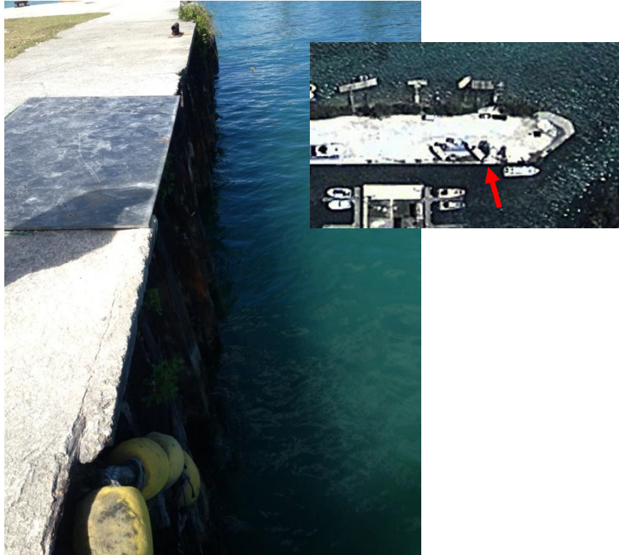
Photo Description: Sheetpile wall along the northern edge of the marina boat basin.
