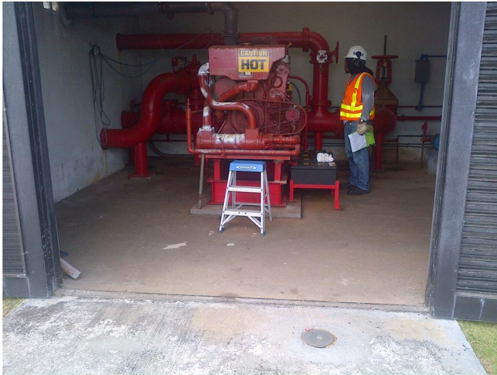
Photo Description: Freshwater fire pump on southern border of Tank Farm A looking north.
