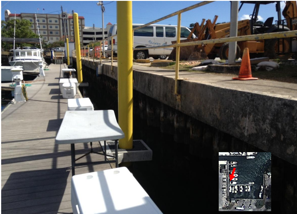
Photo Description: East side of central peninsula looking south. Sheetpile and concrete cap are currently being replaced around southern end of eastern basin.
