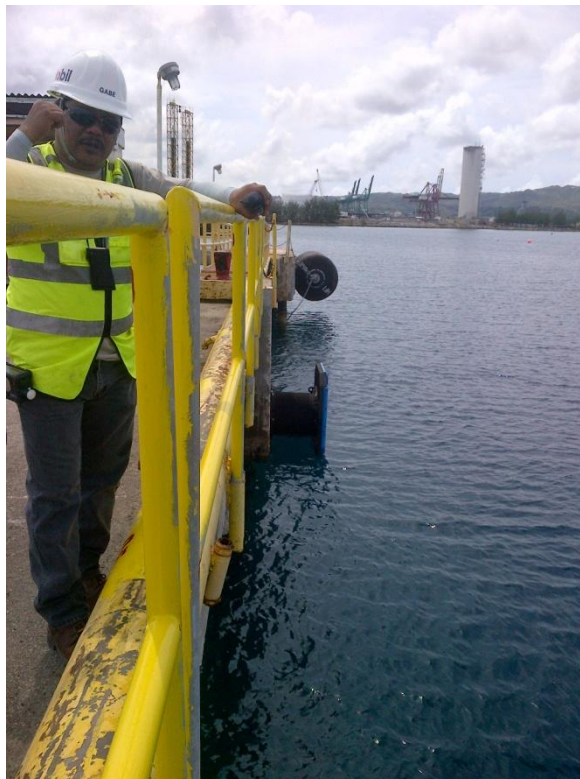
Photo Description: Fenders on the breasting dolphin and eastern end of the Golf Pier main structure looking east.
