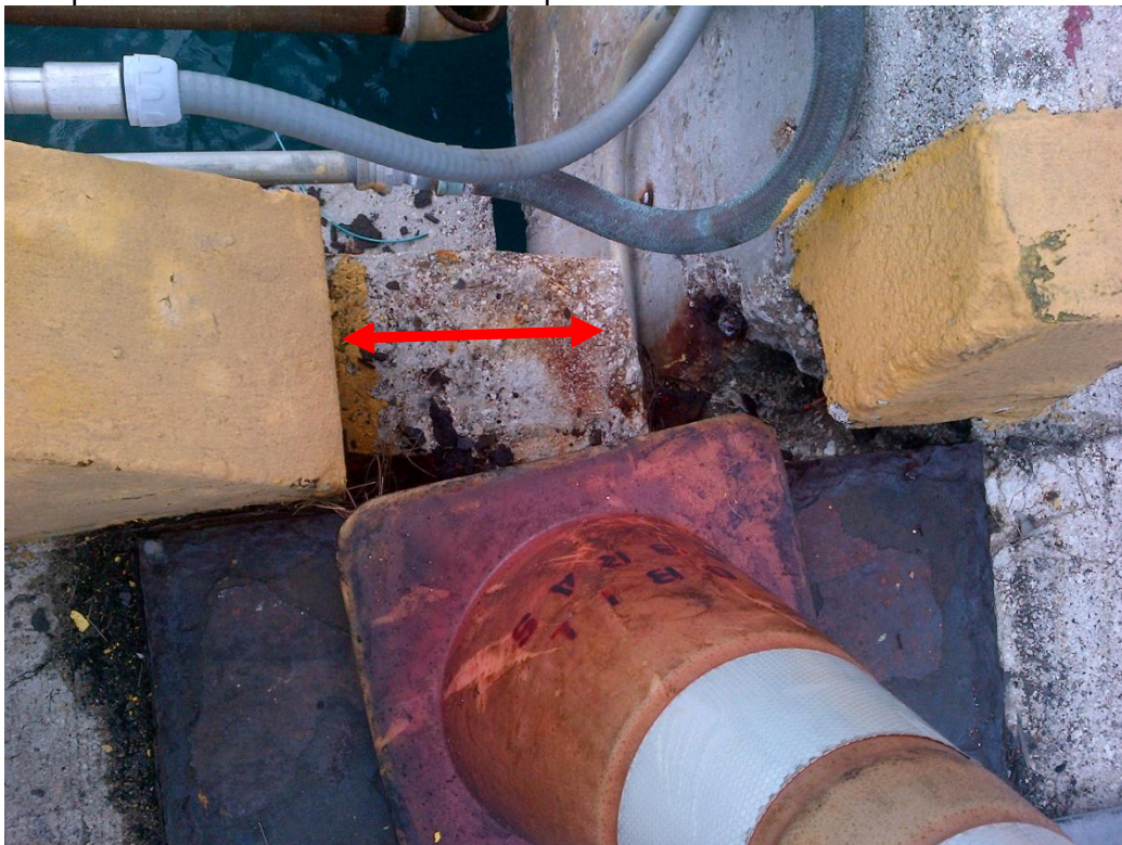
Photo Description: Golf Pier main structure has shifted away from the shore approximately 6-8 inches since originally constructed. As seen on eastern side at pier.
