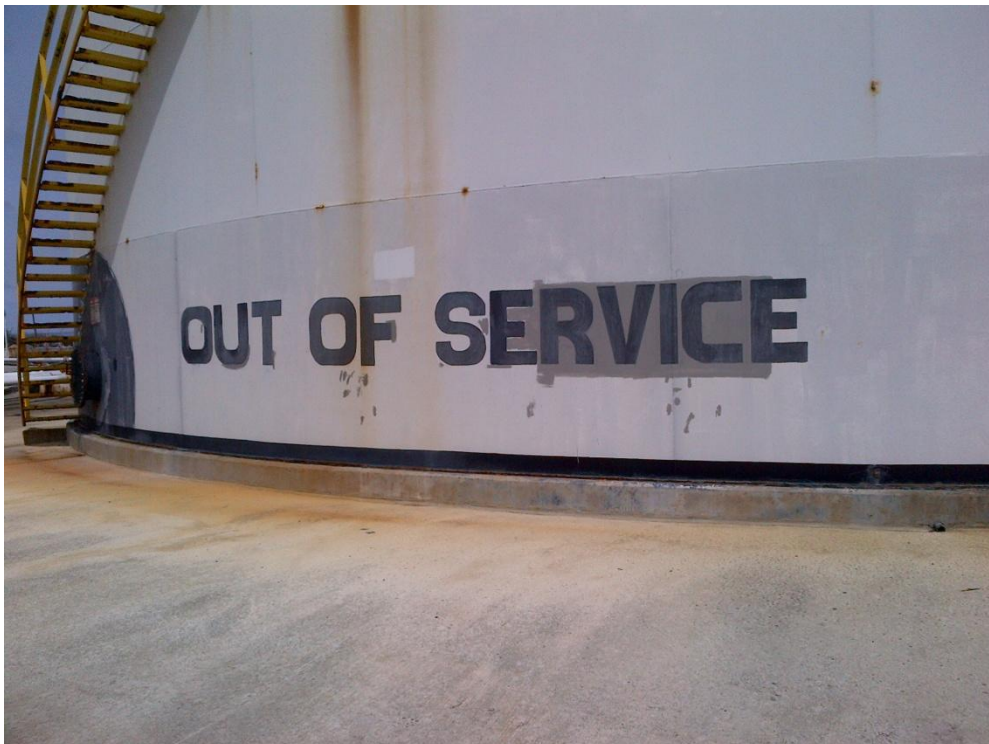
Photo Description: Tank 4 looking from the center of the site to the west. Stairway is in poor condition.
