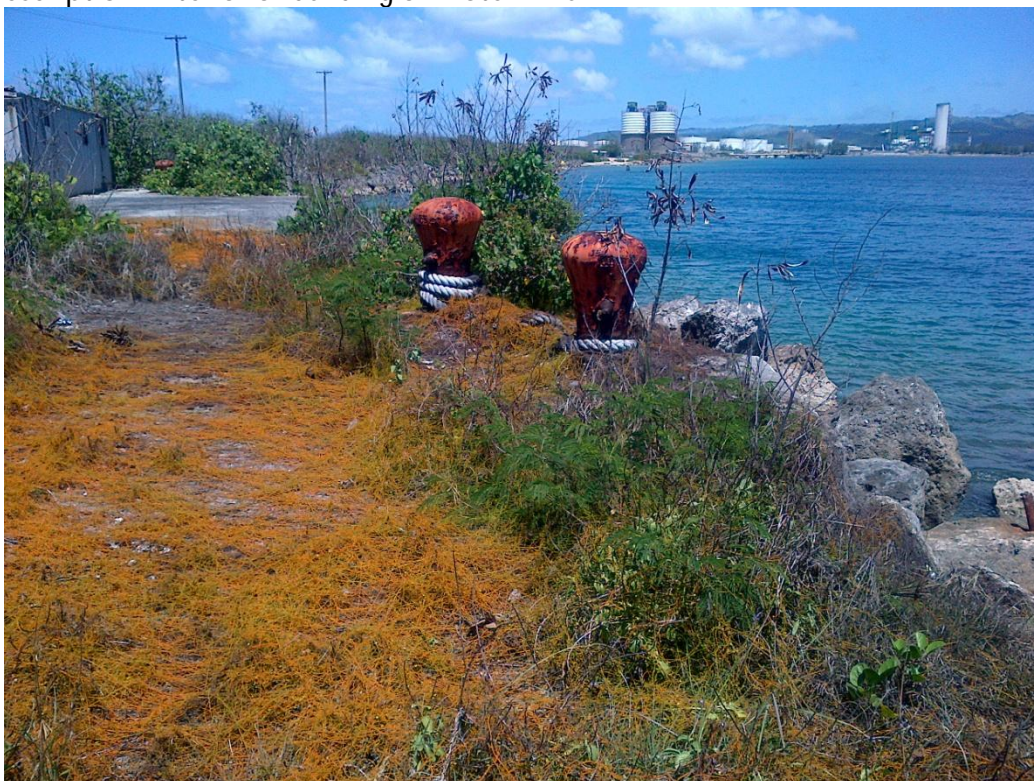
Photo Description: Shoreline bollards east of the wharf structure looking east towards the Main Terminal.
