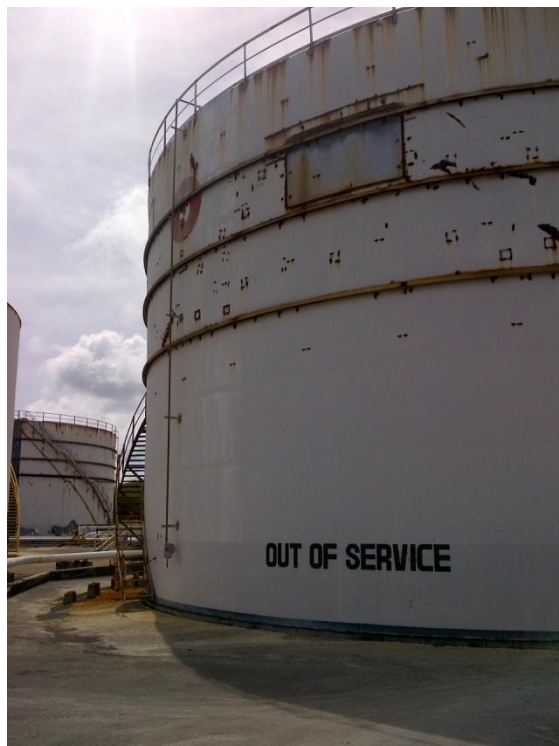
Photo Description: Tank 6 looking east from western ramp. The stairway is unusable in its current state. Tank is out of service.
