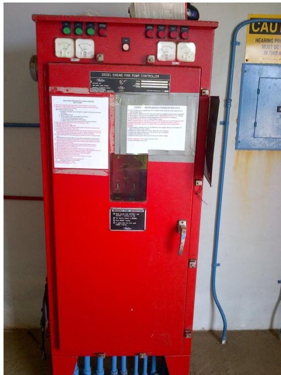
Photo Description: Diesel fire pump control panel in eastern wall of pump building.
