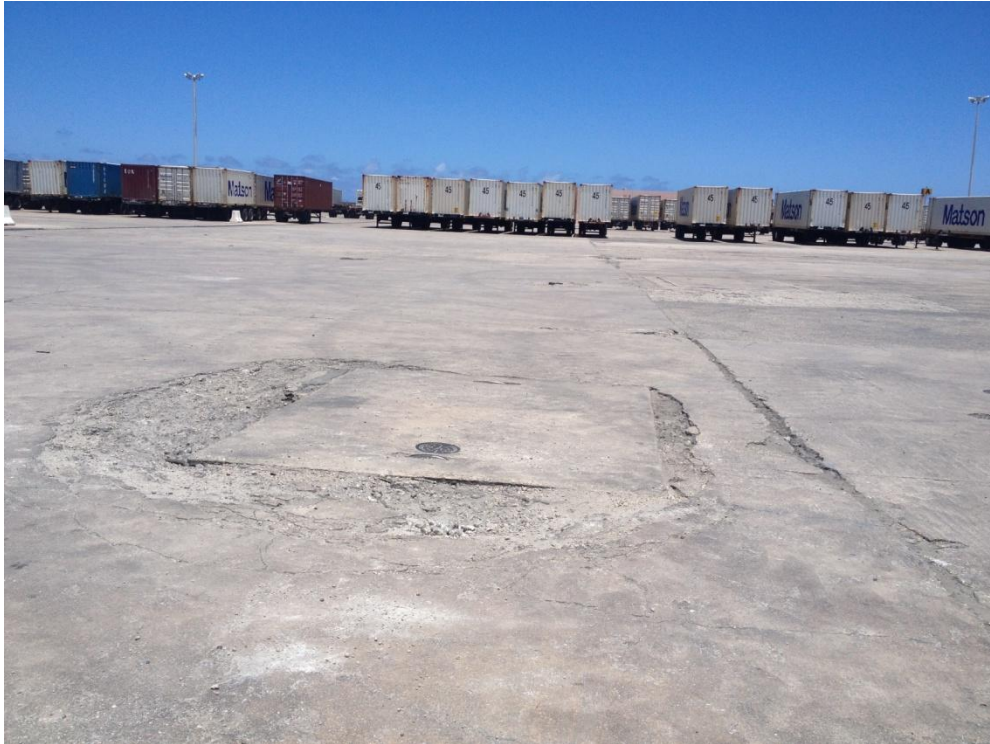
Photo Description: Container yard pavement surface in the 1990 yard expansion. Spalling of the concrete was observed.
