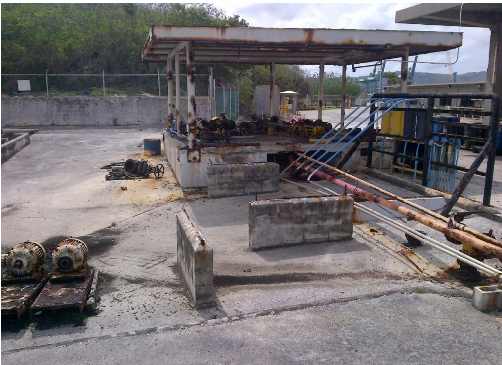
Photo Description: Pump shelter located south of the drum storage looking east. Old valves and components are stored here. The loading rack is to the right of the photo.
