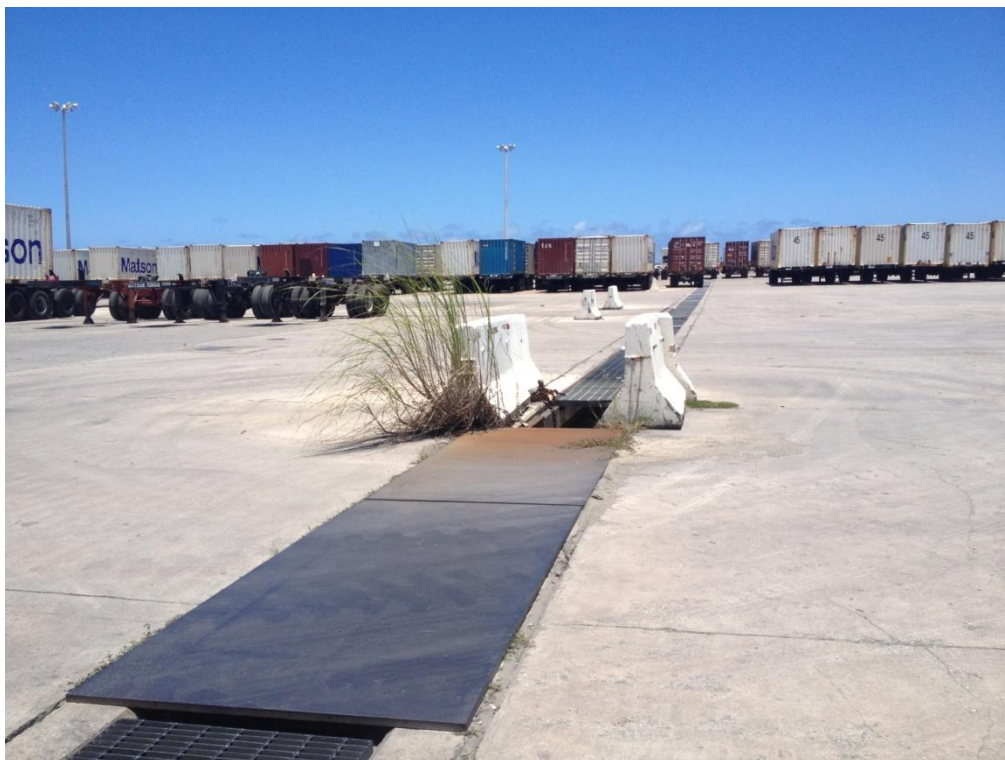
Photo Description: Trench drains on the eastern portion of the yard. The grates and ledges are failing under the loading from the heavy equipment in the container yard.
