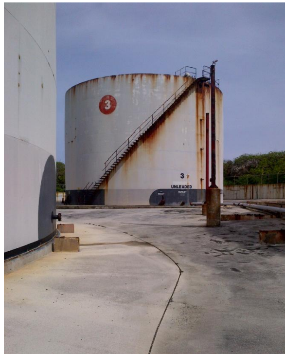
Photo Description: Tank 3 looking from next to tank 4 northwest. The tank has been disconnected and is not in service. The stairway is unusable.
