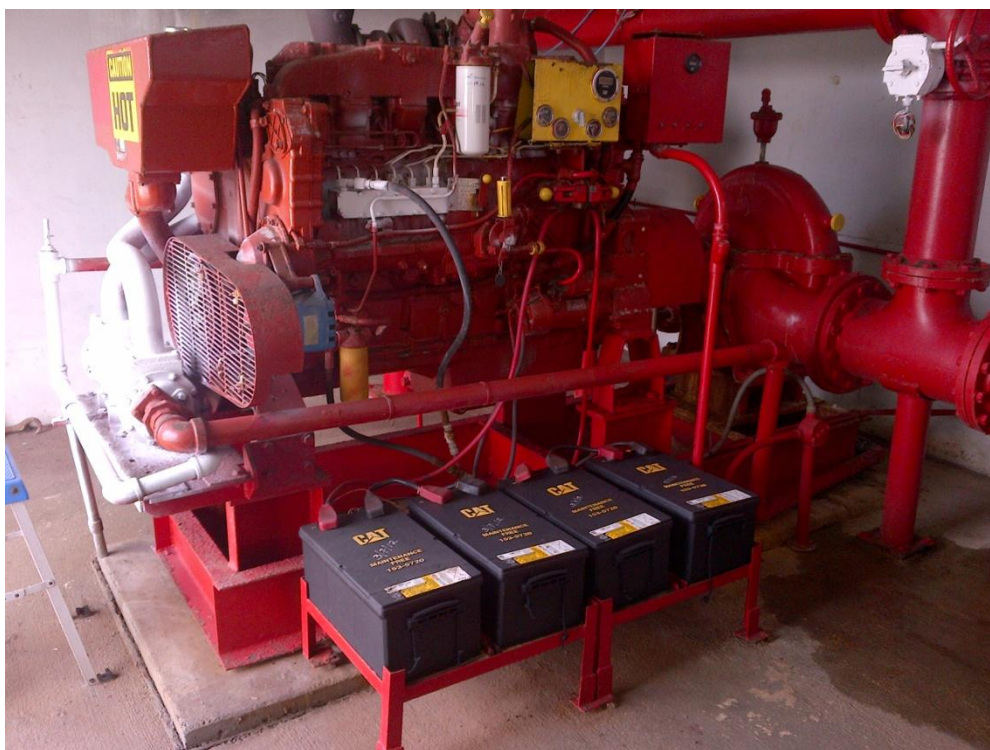
Photo Description: Freshwater fire pump on southern border of Tank Farm A looking northwest.
