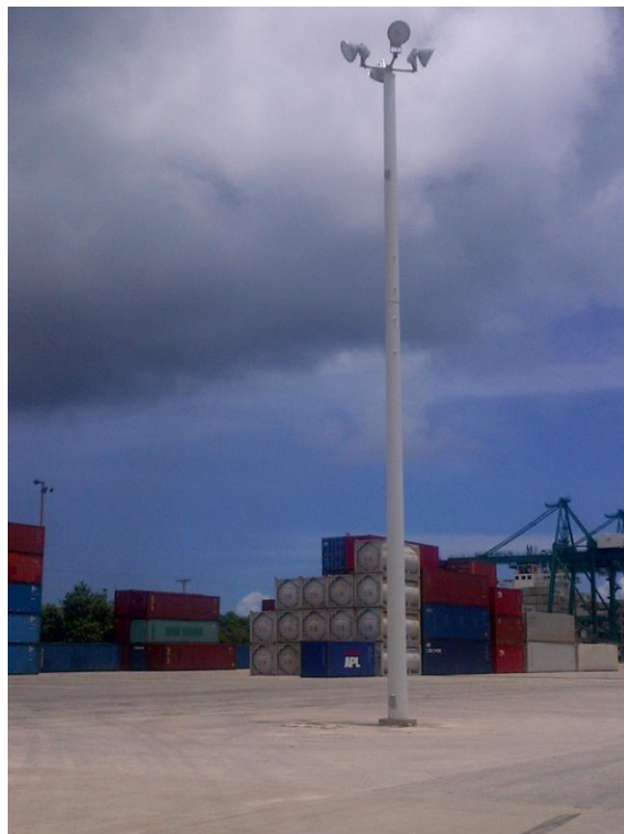
Photo Description: Container yard lights installed in 2012 in the eastern portion of the yard looking southwest.
