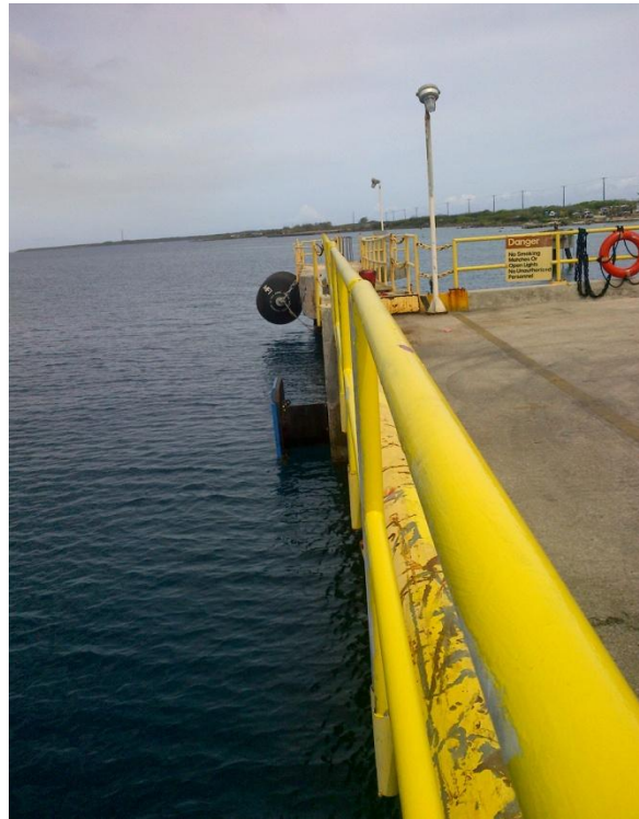
Photo Description: Fenders on the breasting dolphin and western end of the Golf Pier main structure looking west.
