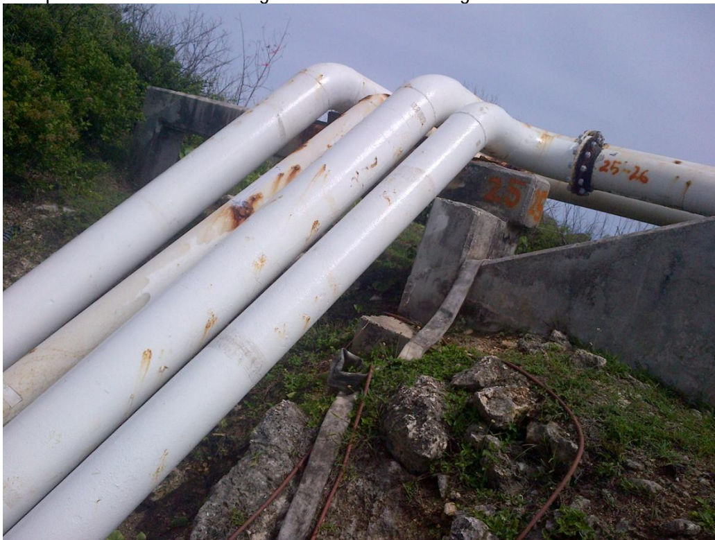
Photo Description: Fuel lines on the north side of the access road. The pipes are elevated on the north side of the road as they continue to Tank Farms A and C.
