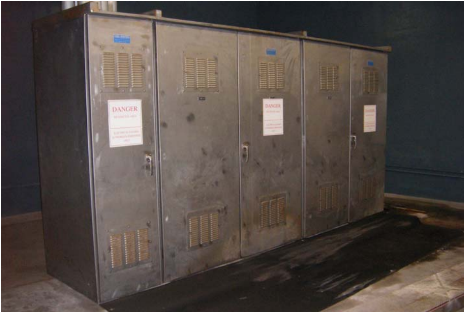
Photo description: Stainless steel Switchgear and transformer in LC-4
