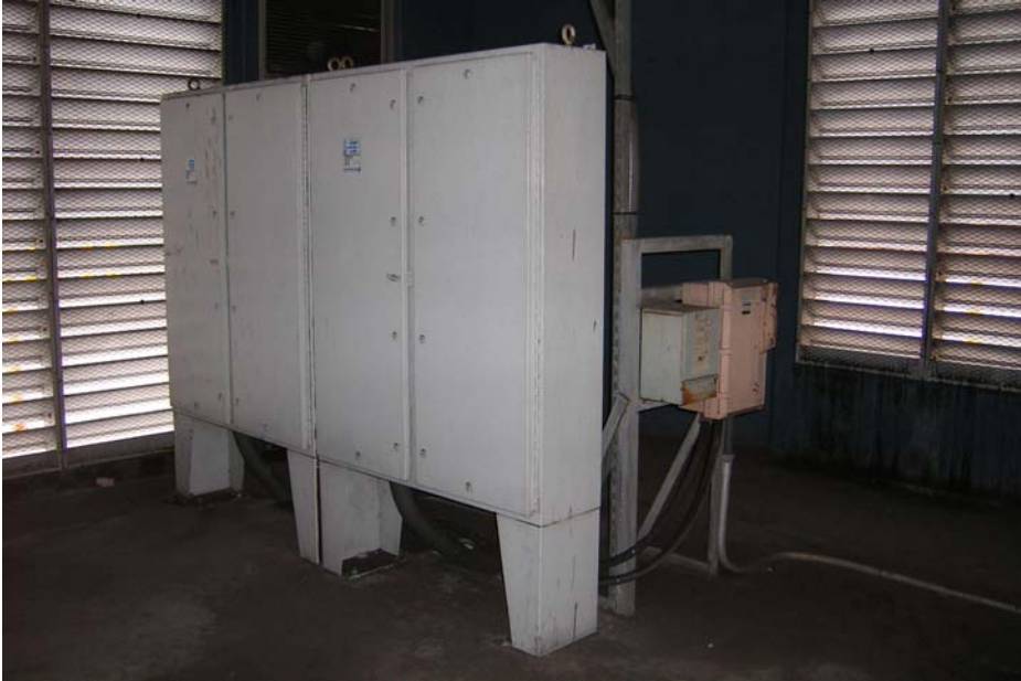
Photo description: Cathodic protection panel in LC-3
