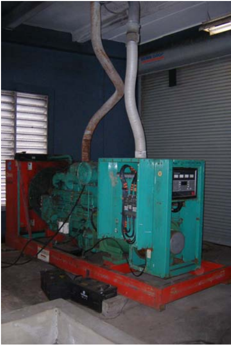
Photo description: Emergency generator in LC-3
