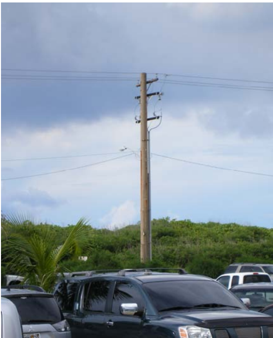
Photo description: GPA lead in light pole
