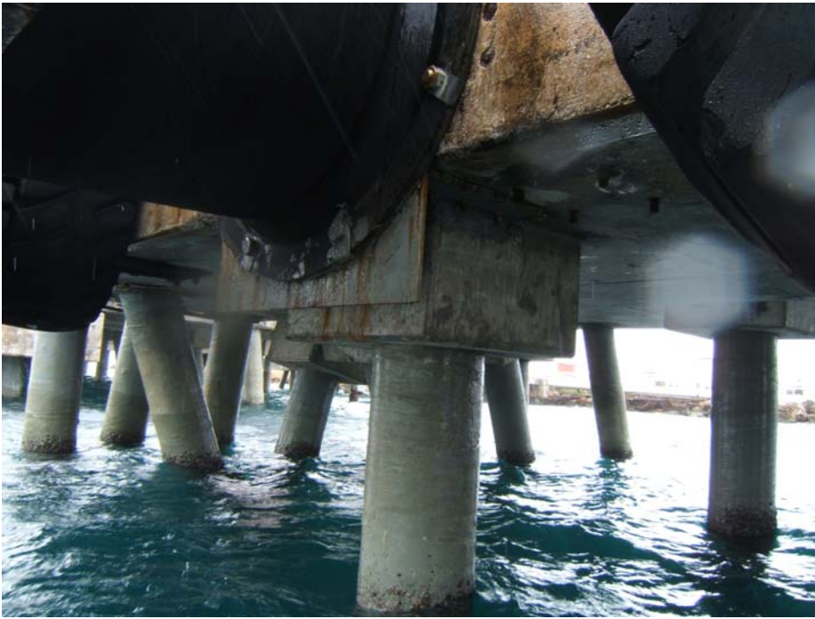
Photo description: steel pile for F-1 deck, retrofit to earthquake damage on top portion
