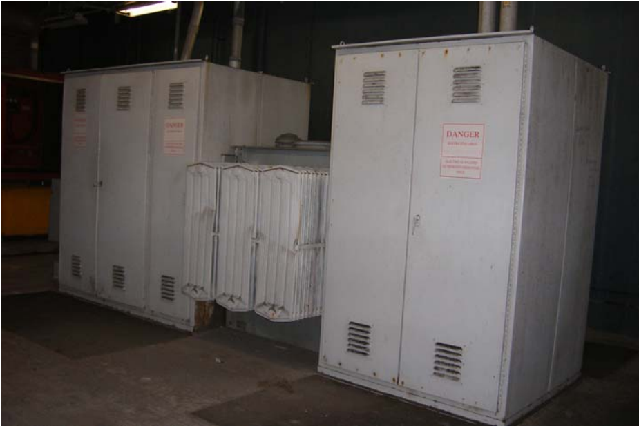
Photo description: Switchgear and transformer in LC-2
