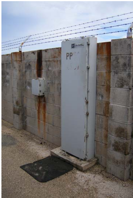
Photo description: Power panel supplying the reefer outlets
