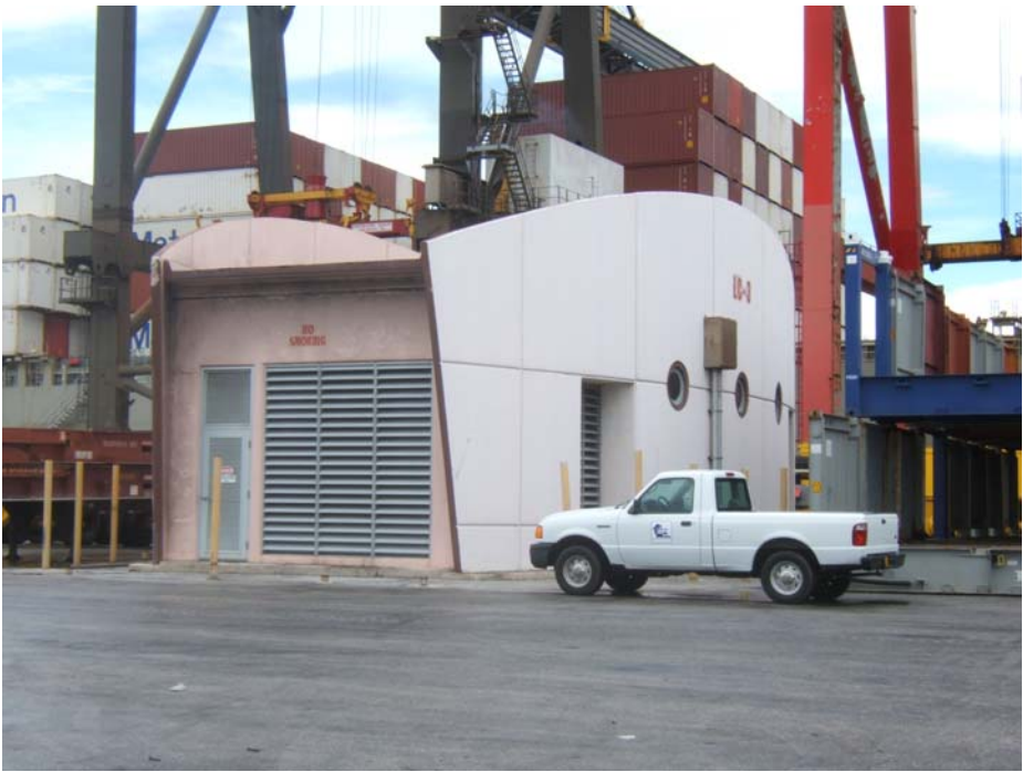
Photo description: Load Center (LC #3)
