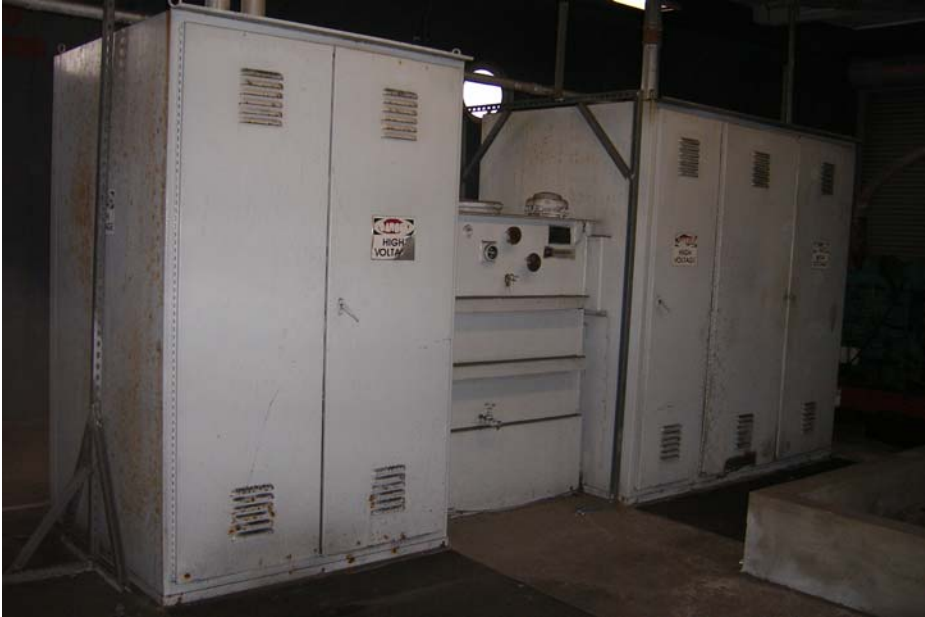
Photo description: Switchgear and transformer in LC-3
