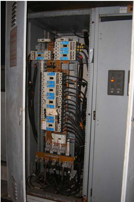
Photo description: Inside view of power panel in LC-2
