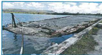
Submerged Barge at Wharf F6
