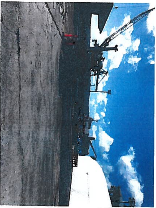
Existing 4,000 Gallon Diesel Fuel Tank
