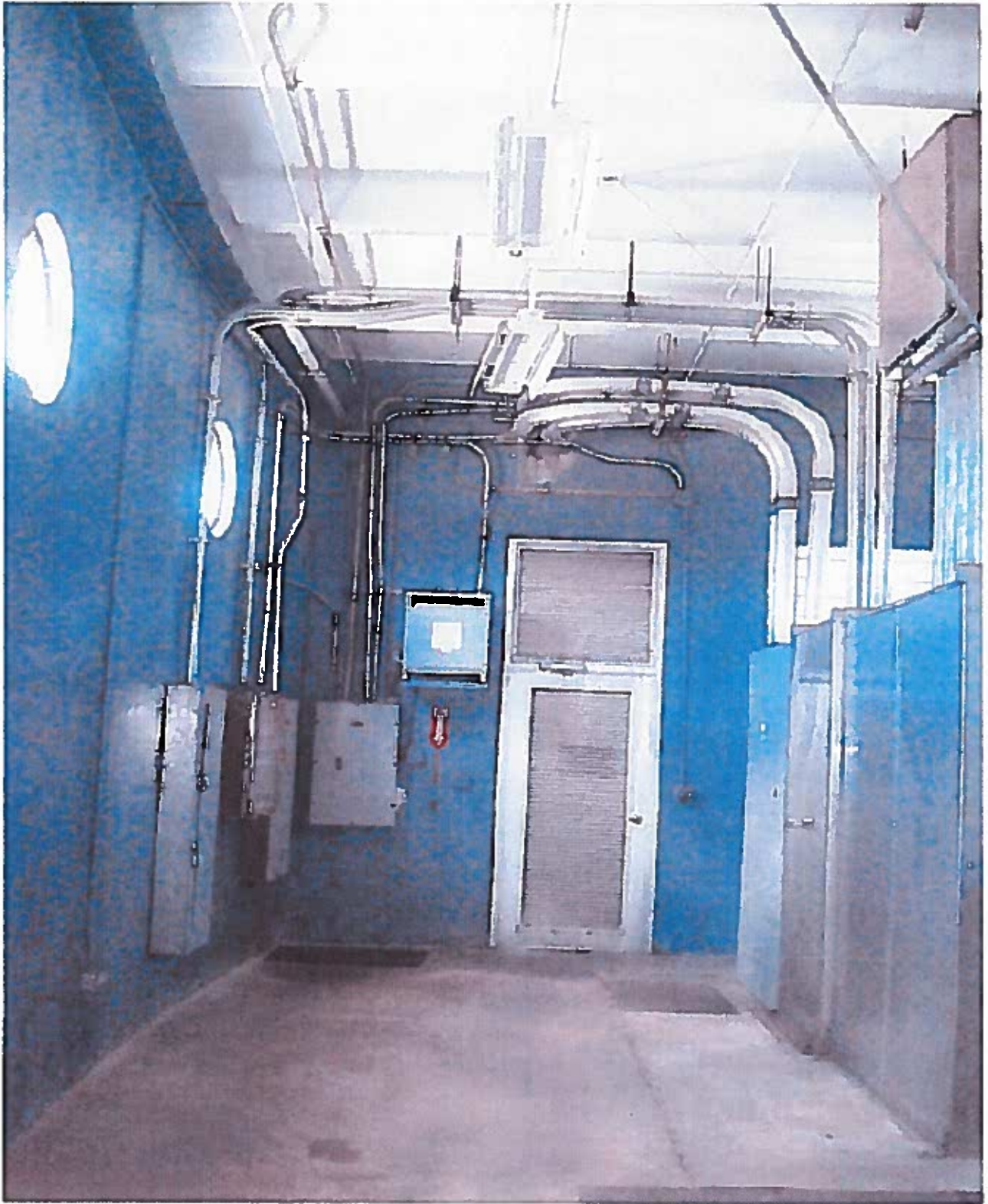
LC-1 INSIDE ELECTRIC BREAKERS AND PANELS
