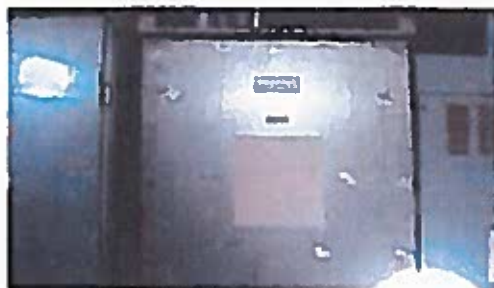
STREET LIGHT PANEL
