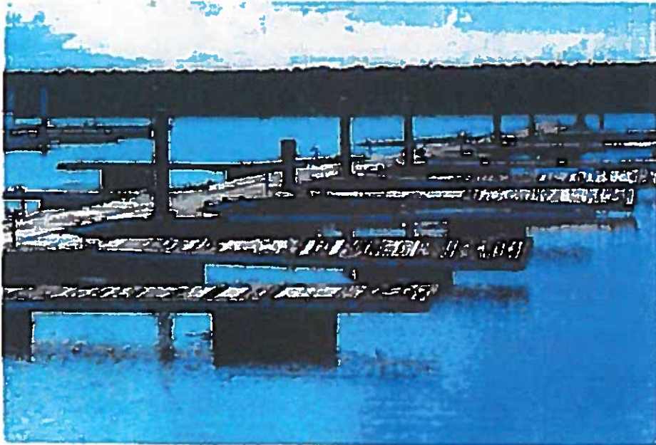
View of condemned Dock B (to be removed and replaced).
